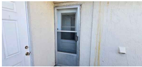
Unprotected glazed entry doors
