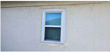
Unprotected glazed openings
