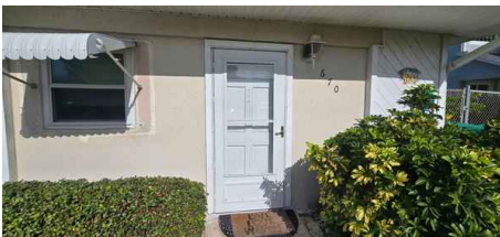
Unprotected non-glazed entry door
