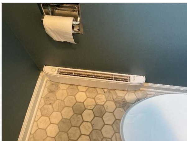
Baseboard heater 1st floor 1/2 bath
