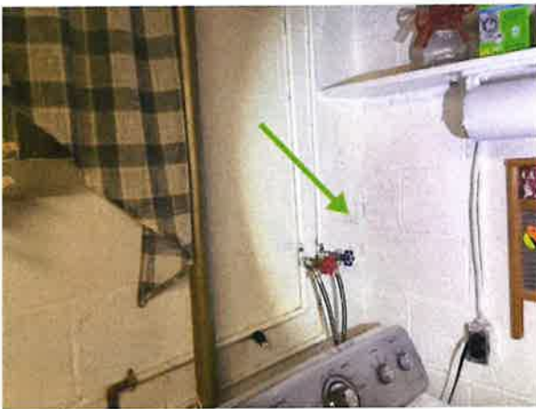
Laundry room left rear
