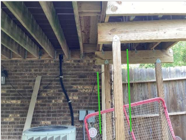
Vertical post do not appear plumb
