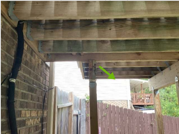
Header not plumb
