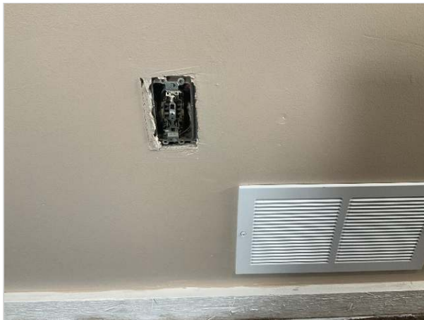
Live outlet noted in master bedroom
