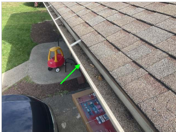
shingle aggregate debris noted in gutters
