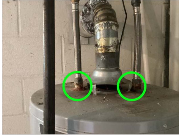
Evidence of corrosion
