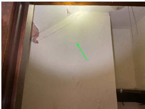
detection area - front chimney
