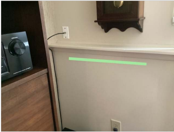
Area of high moisture
