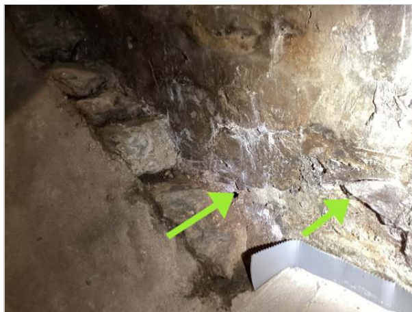
Open mortar and crack
