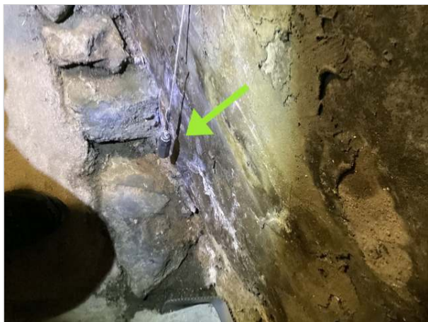
Approximately 2 inch offset
