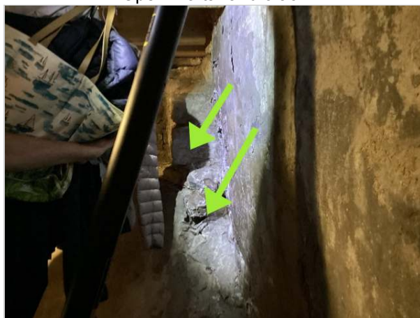
Evidence of deterioration
