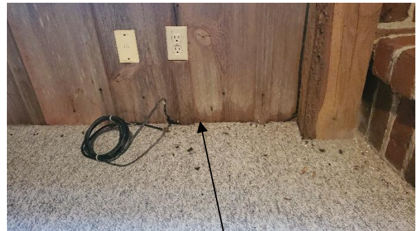
West wall – water damage
