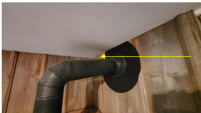
Too close to ceiling
