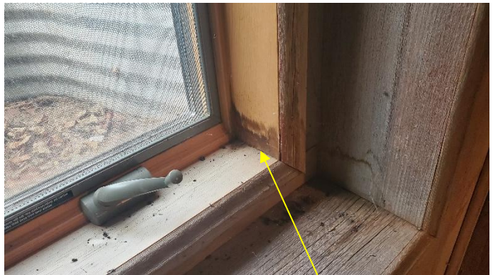
Water stained window
