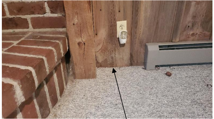
North wall – water stained
