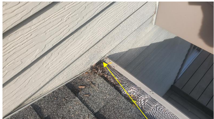
No kickout flashing
