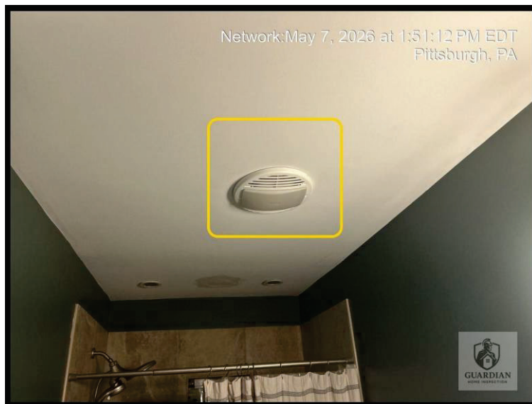
Figure 8: The light bulb in the second-floor bathroom exhaust fan/light fixture was reported as inoperable.
