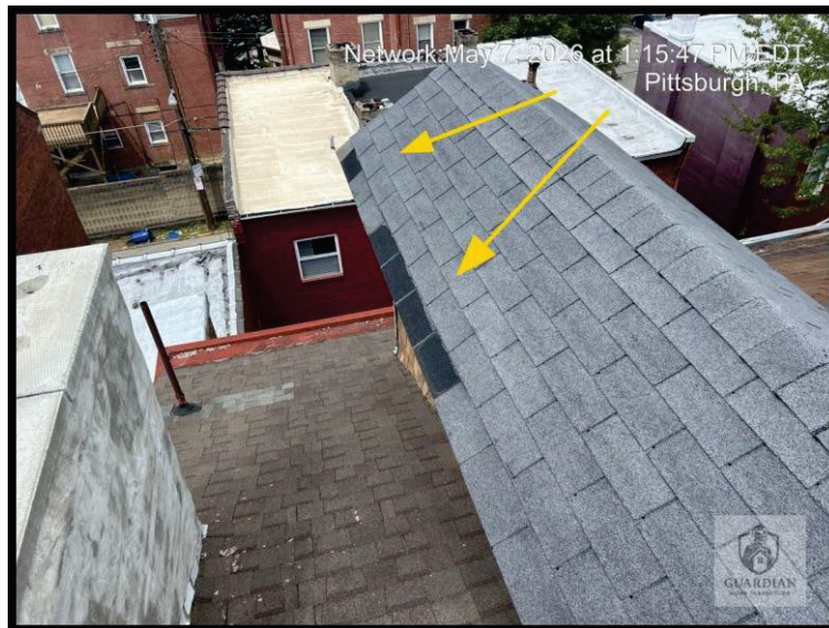
Figure 5: Several asphalt shingles were observed missing on the rear-facing dormer roof.
