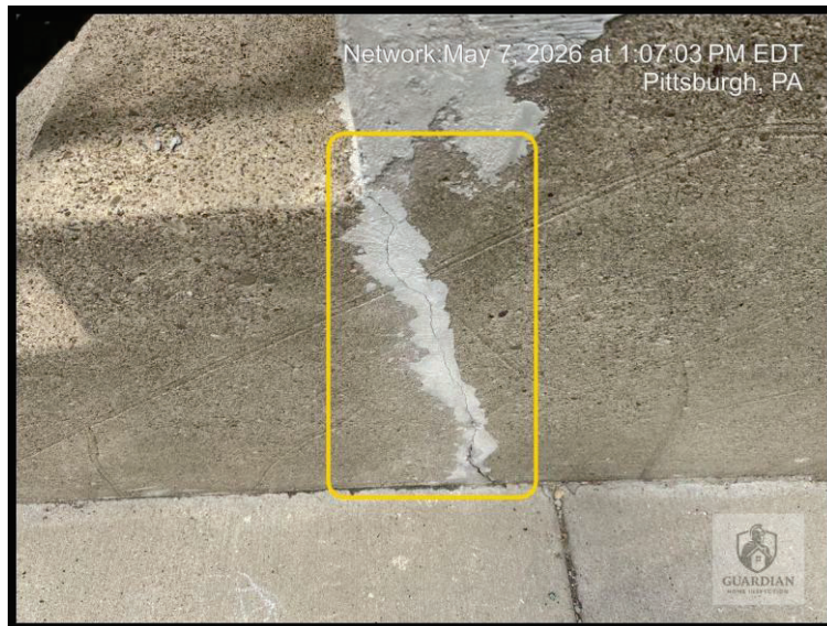
Figure 11: The front-facing porch/stoop exhibited evidence of minor cracking.
