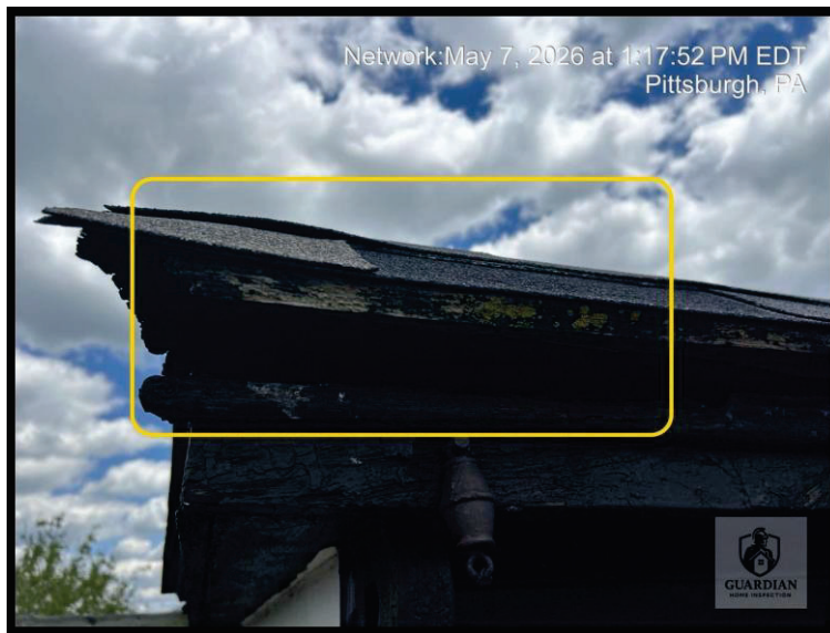
Figure 2: The rear-facing dormer exhibited evidence of wood rot along the eave, with deteriorated/decayed wood visible at the trim/soffit area.
