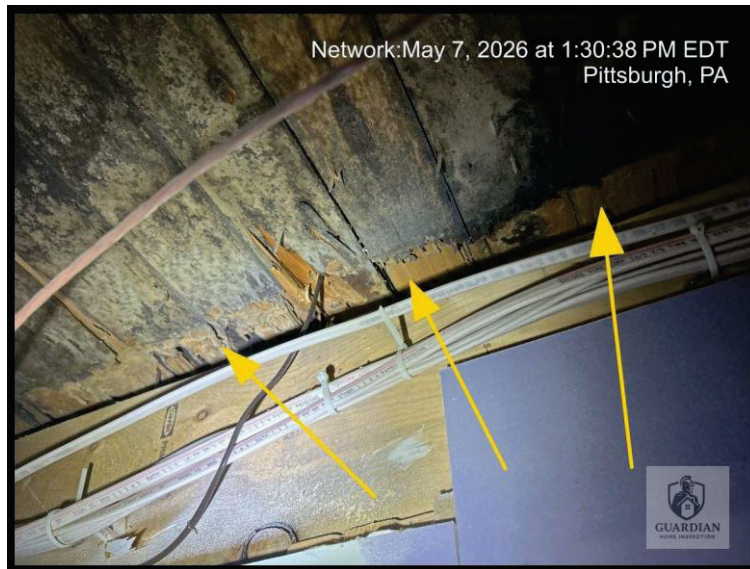
Figure 9: Termite-related damage was observed along the subfloor above the center basement wall; the visible activity appeared inactive at the time of inspection.
