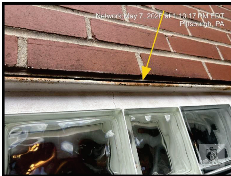
Figure 12: Steel lintels at the exterior masonry opening were observed with exposed metal and surface rust staining.
