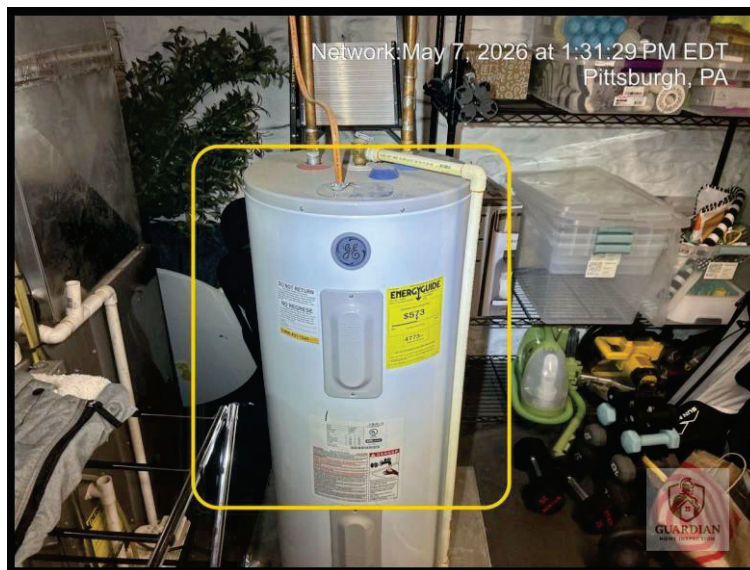
Figure 14: The basement water heater was observed to be approaching the end of its typical useful life for similar units.
