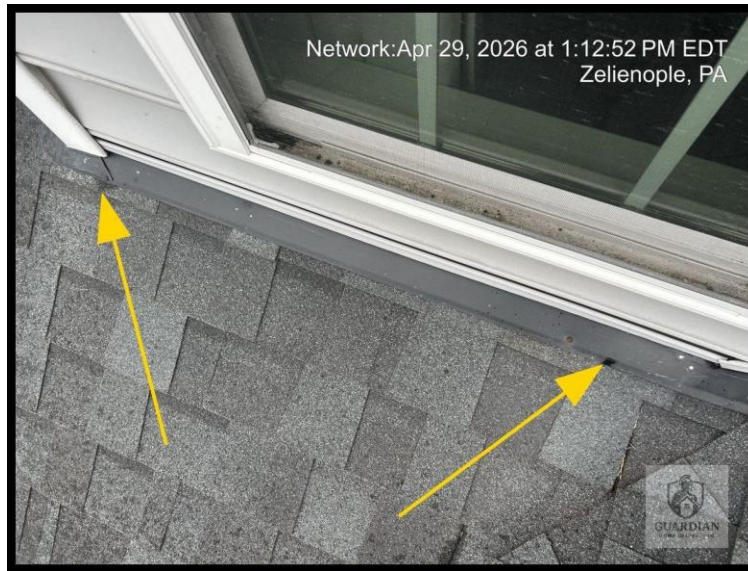
Figure 7: Roof-to-wall flashing and diverter flashing at the roof area were observed with exposed nail heads that require sealing, as visible at the flashing edges.
