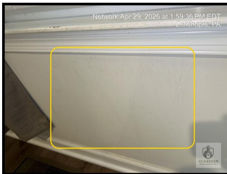
Figure 17: Minor damage/scuffing was observed on the drywall finish along the second-floor front-facing windows in the loft area (hallway).
