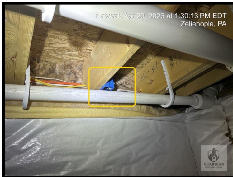
Figure 1: An open electrical junction box was observed along the basement ceiling.
