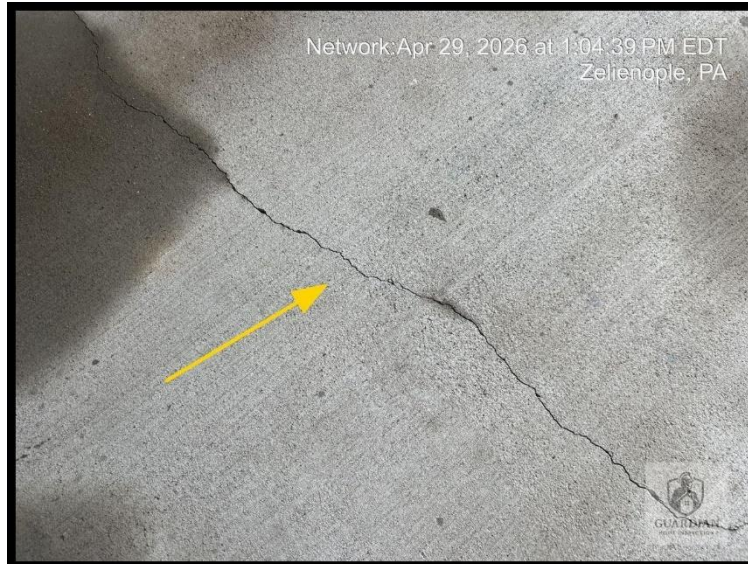
Figure 5: Minor cracking was noted along the rear patio concrete slab.
