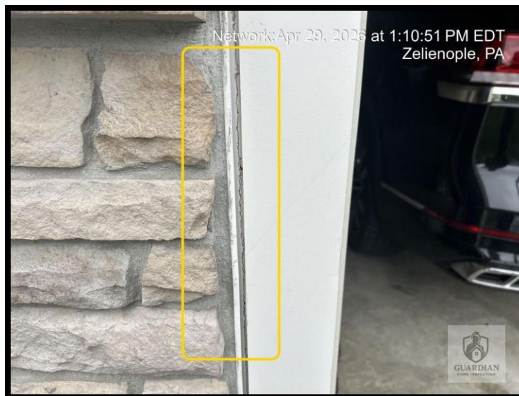
Figure 6: Exterior window and door frames/trim were observed with areas needing resealing and caulking (notably at trim-to-masonry/trim joints).
