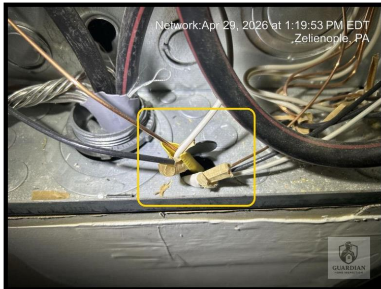
Figure 9: In the garage, electrical conductors were observed passing through the main electrical panel cabinet without an approved protective cable clamp/bushing at the cabinet knockout.
