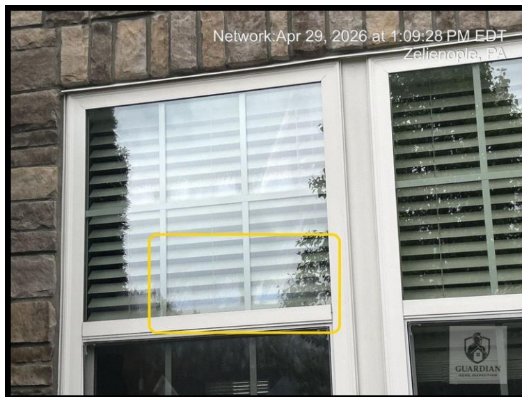
Figure 12: The front-facing first-floor window in the Family Room was observed to be fogged, consistent with moisture between the panes of an insulated glass unit.
