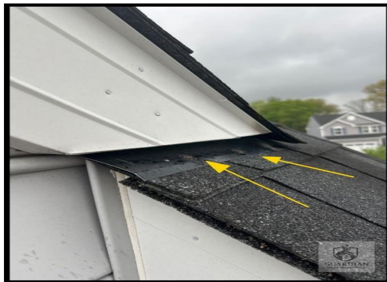
Figure 8: Roof-to-wall flashing and diverter flashing at the roof area were observed with exposed nail heads that require sealing, as visible at the flashing edges.
