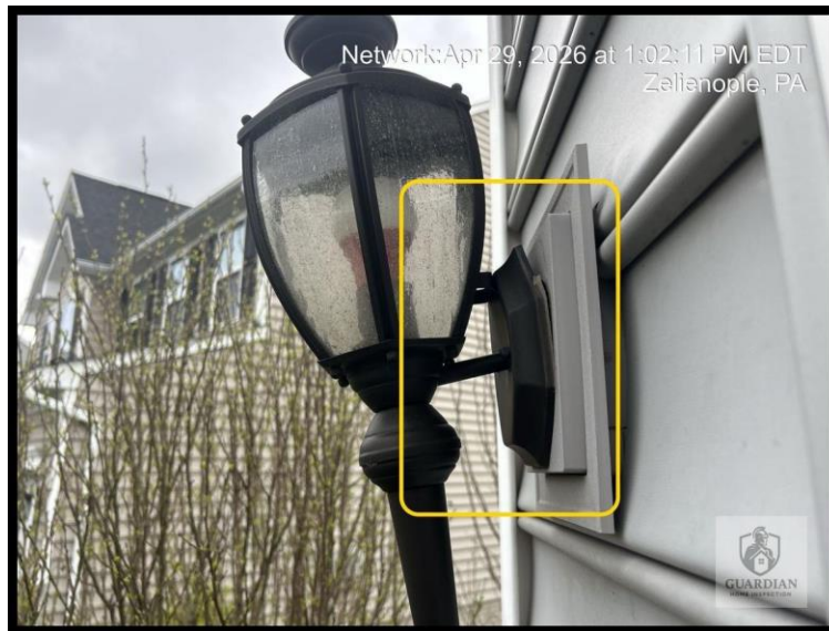
Figure 3: The front-facing exterior light fixture housing was observed to be loose from the wall.
