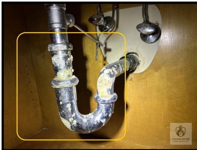
Figure 12: The drain piping (P-trap assembly) under the hallway bathroom sink was observed to be severely pitted/corroded.
