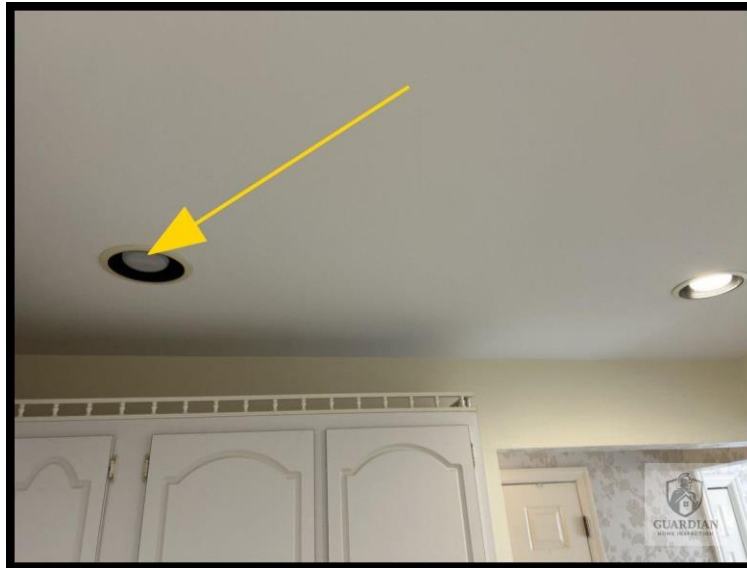
Figure 3: Several light bulbs were observed to be blown/non-functional at light fixtures in the living room, bathroom, and kitchen.
