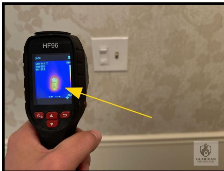
Figure 16: The dining room chandelier dimmer switch exhibited evidence of overheating when evaluated with a thermal camera.
