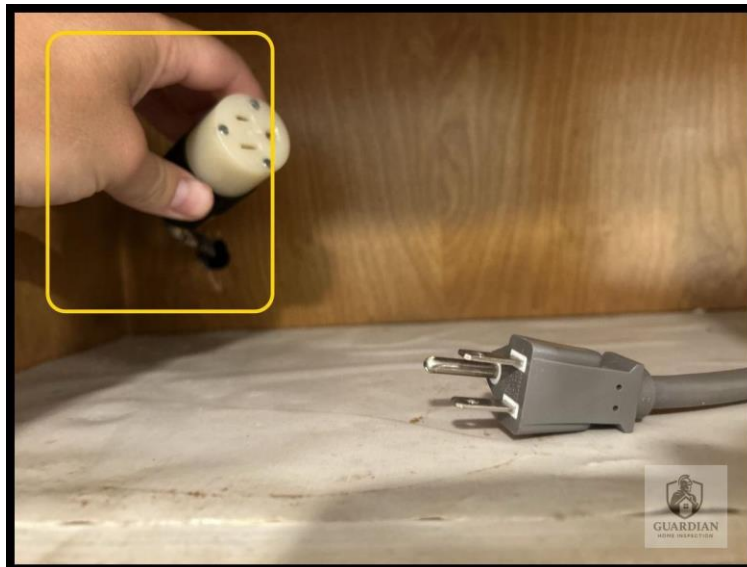
Figure 1: In the kitchen, NM (Romex) cable was observed spliced directly into an extension-cord style plug serving the microwave, which is an improper use of permanent wiring and indicates a noncompliant cord connection.
