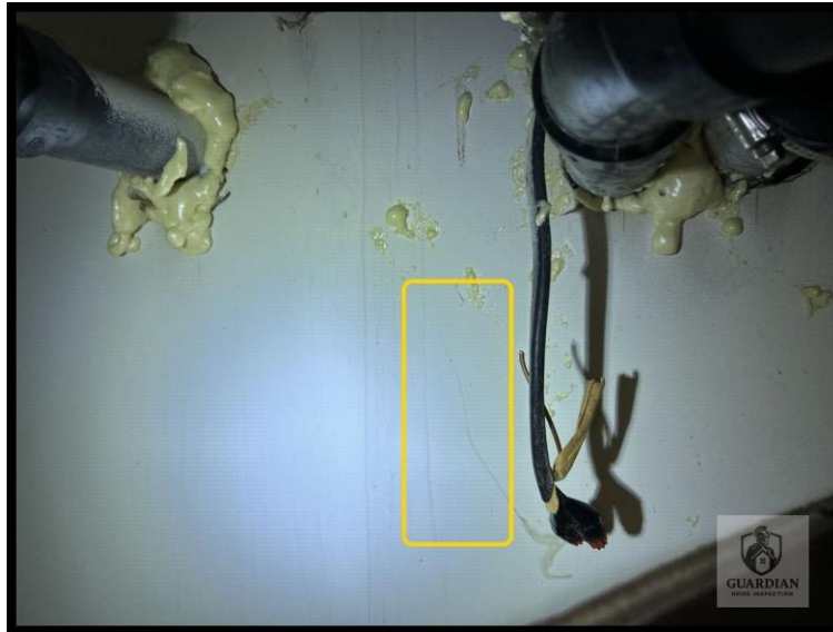
Figure 7: In the kitchen, abandoned electrical wiring reportedly for a waste disposal was observed hanging loose and not properly terminated within an approved junction box.
