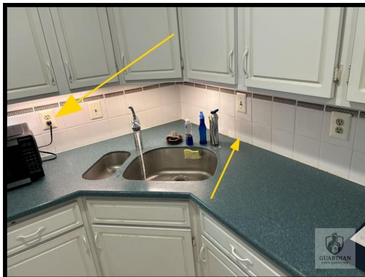
Figure 2: Kitchen countertop receptacles were observed without GFCI protection.
