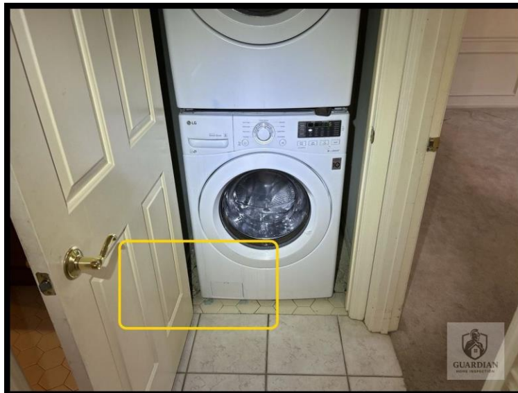
Figure 22: A catch pan was not observed under the clothes washer in the laundry room.
