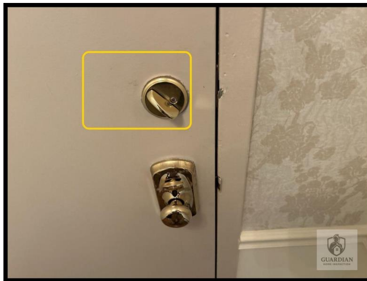
Figure 23: The main entry door deadbolt at the living room would not fully lock/engage during operation.
