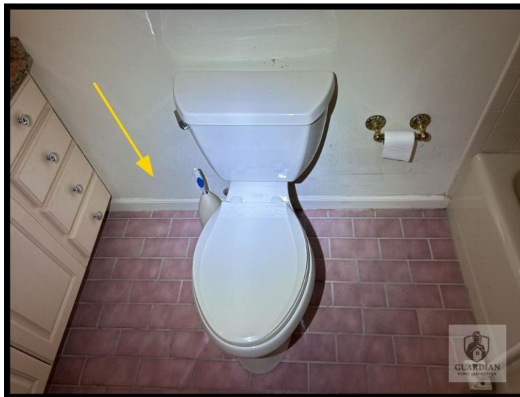
Figure 10: The toilets observed in the bathrooms were loose at the floor attachment.
