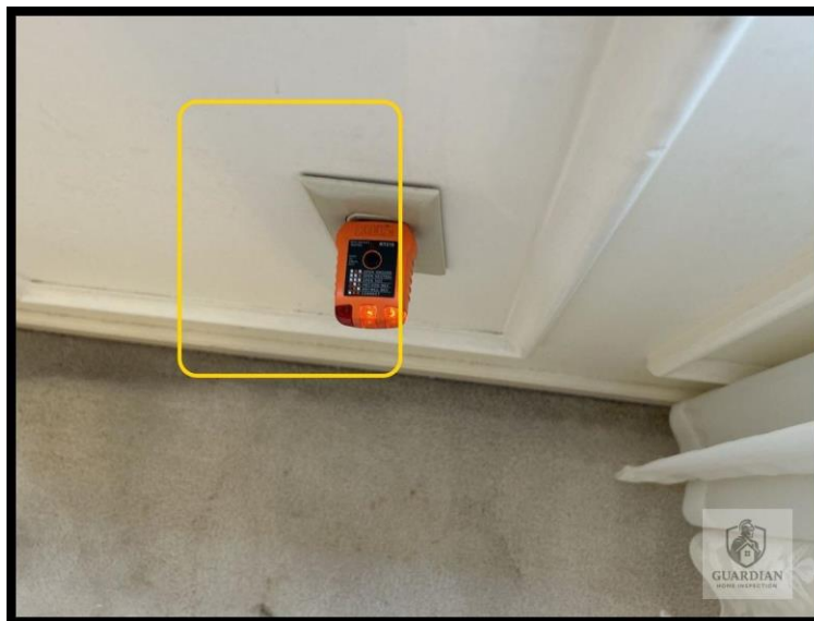
Figure 20: Several electrical outlets were observed to be loose from the wall in the Bedroom and Kitchen; the pictured receptacle plate appears not securely seated/flush to the wall surface.
