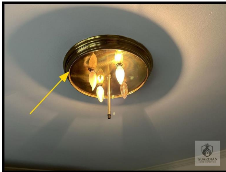
Figure 4: Several light bulbs were observed to be blown/non-functional at light fixtures in the living room, bathroom, and kitchen.
