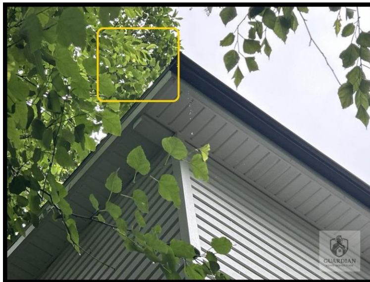
Figure 10: Several gutter corner seams at the roofline were observed leaking at the time of inspection.
