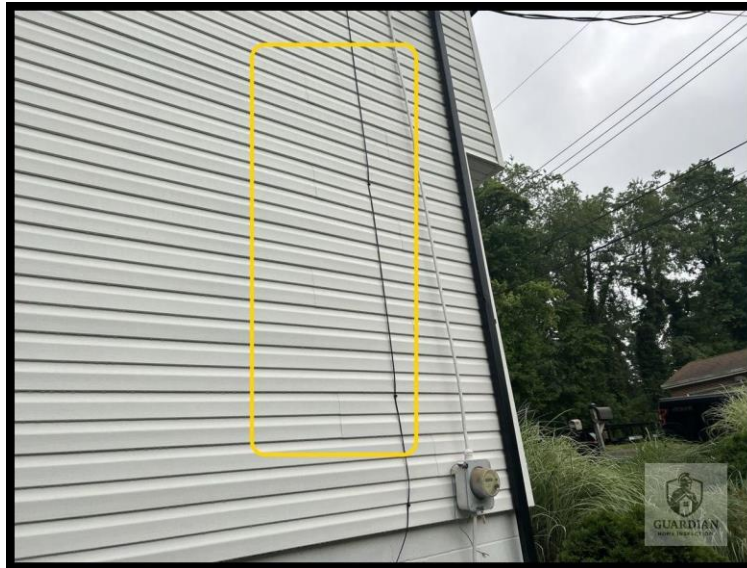
Figure 17: The electrical service cable along the left-facing exterior side of the home was observed to be loose and not adequately secured to the wall.
