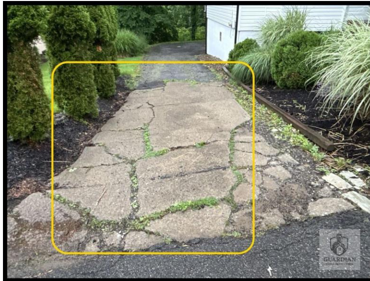
Figure 7: The concrete and asphalt driveway was observed to be in poor condition with widespread cracking, deteriorated/patched areas, and uneven surfaces.
