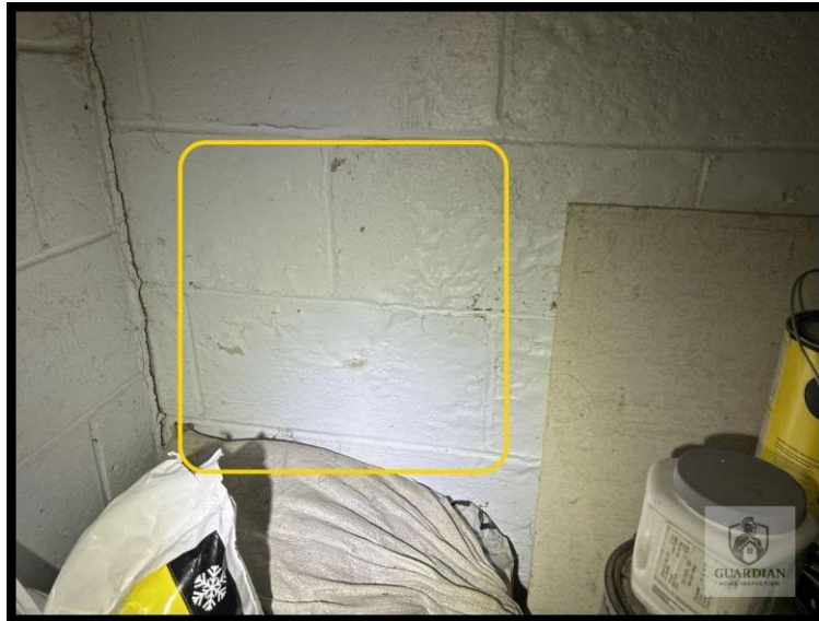
Figure 15: Moisture intrusion was noted along the front-facing basement foundation wall, with visible staining/efflorescence on the masonry surface.
