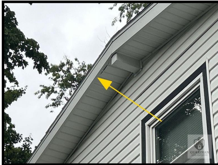
Figure 25: A minorly loose soffit piece was observed along the left exterior eave.
