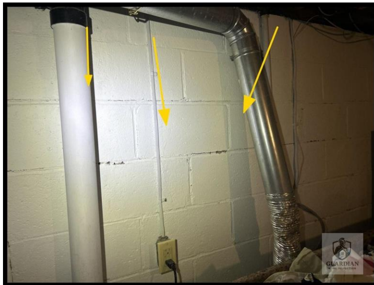
Figure 14: Moderate step and horizontal cracking was observed along the front-facing foundation wall in the basement, as shown in the photos.
