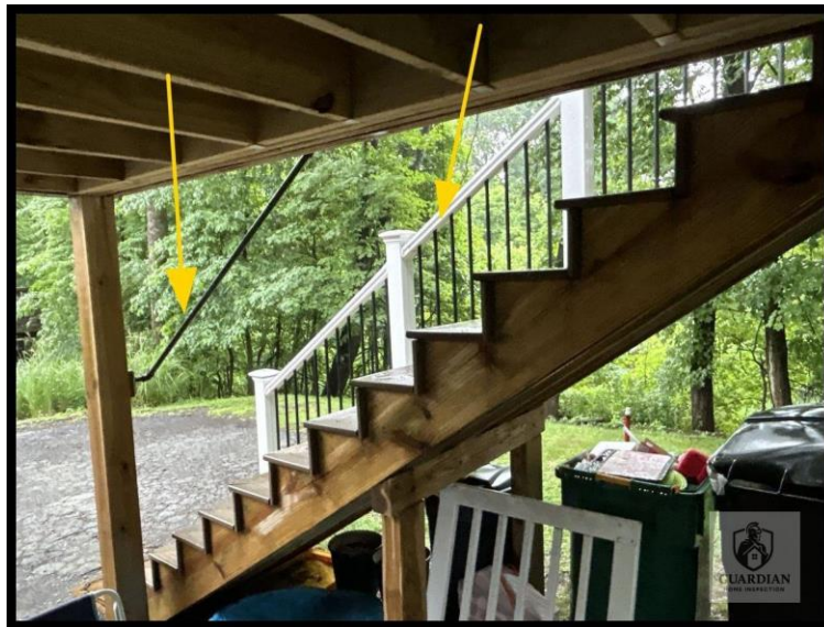
Figure 1: The rear exterior deck stairway has an open side where a step railing/handrail is not installed.
