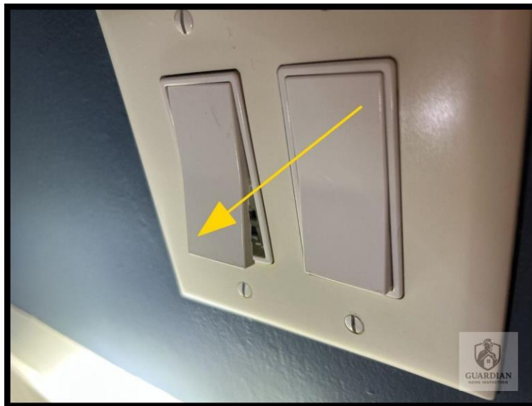
Figure 18: A switch in the first-floor powder room bathroom was observed to be damaged, with a broken/loose rocker visible at the switch opening.
