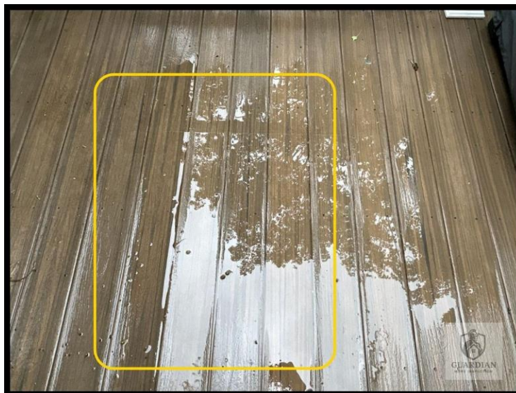
Figure 8: Inadequate spacing was observed along the rear exterior deck planking.
