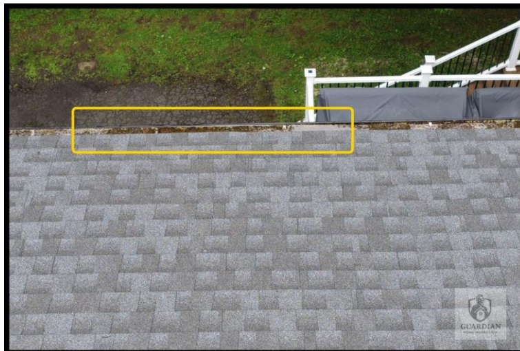
Figure 12: The roof gutters were observed to be full of debris and spilling over along the eaves.
