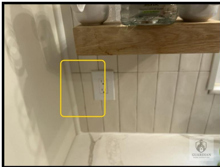
Figure 2: A receptacle located along the kitchen countertop was observed without GFCI protection.
