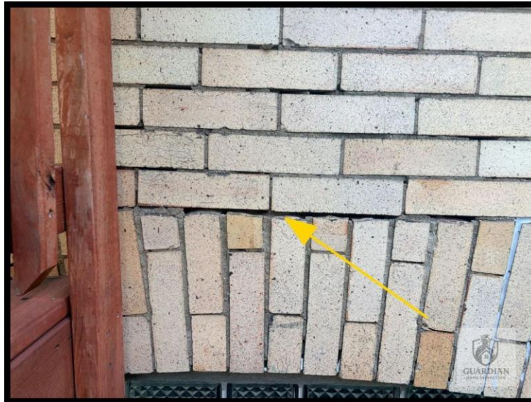
Figure 21: Stepped cracking and mortar joint separation were observed in the exterior brick veneer, consistent with possible building movement/settlement.
