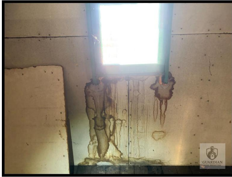
Figure 27: Significant water intrusion staining and damaged sheathing/drywall were observed in the attic around the chimney and a window, with evidence consistent with a past leak.
