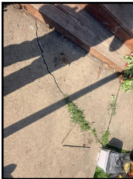
Figure 4: Cracked and broken concrete was observed at the exterior walkway/landing, with vegetation growth through the damaged areas and resulting uneven surfaces.
