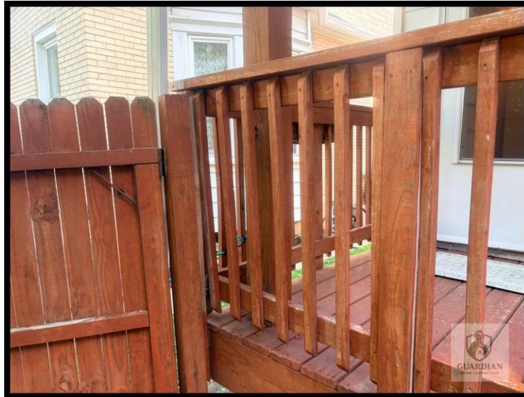
Figure 7: A loose hand railing was observed at the rear porch.
