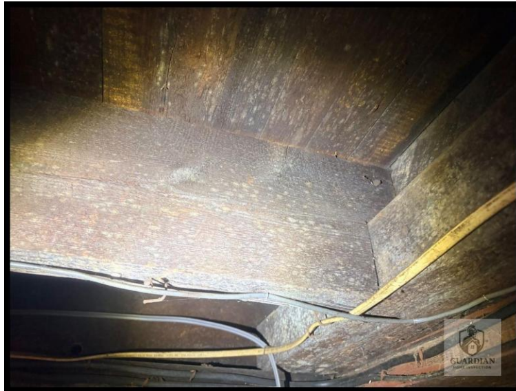
Figure 3: Over-notched and poorly constructed floor joists were observed in the basement.
