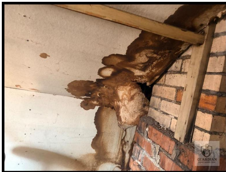
Figure 26: Significant water intrusion staining and damaged sheathing/drywall were observed in the attic around the chimney and a window, with evidence consistent with a past leak.
