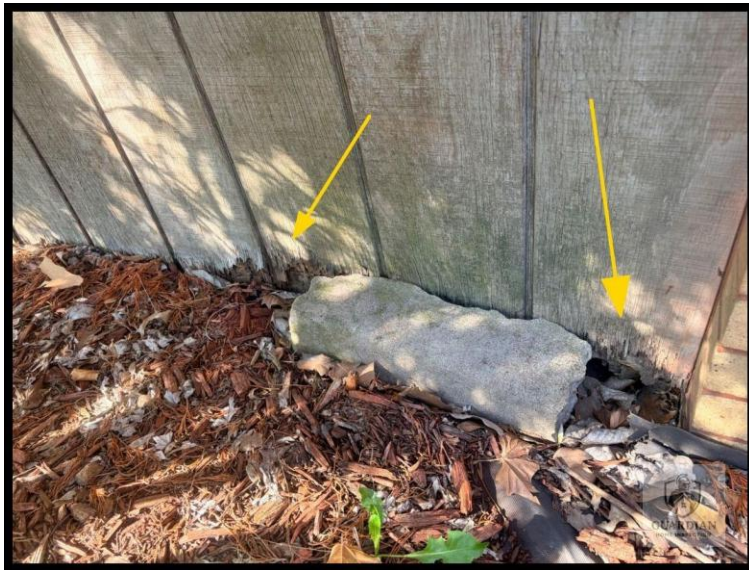
Figure 14: Rotted and deteriorated wood siding was observed at the bottom edge at the exterior, with a visible gap/opening at the base.
