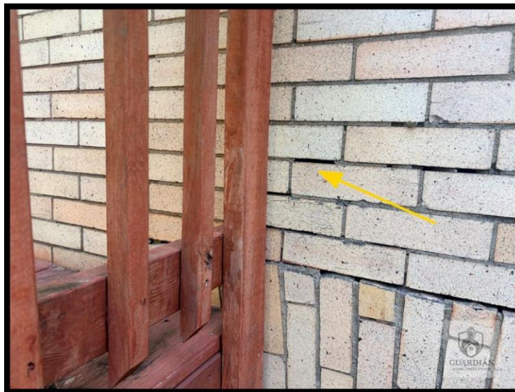
Figure 22: Stepped cracking and mortar joint separation were observed in the exterior brick veneer, consistent with possible building movement/settlement.
