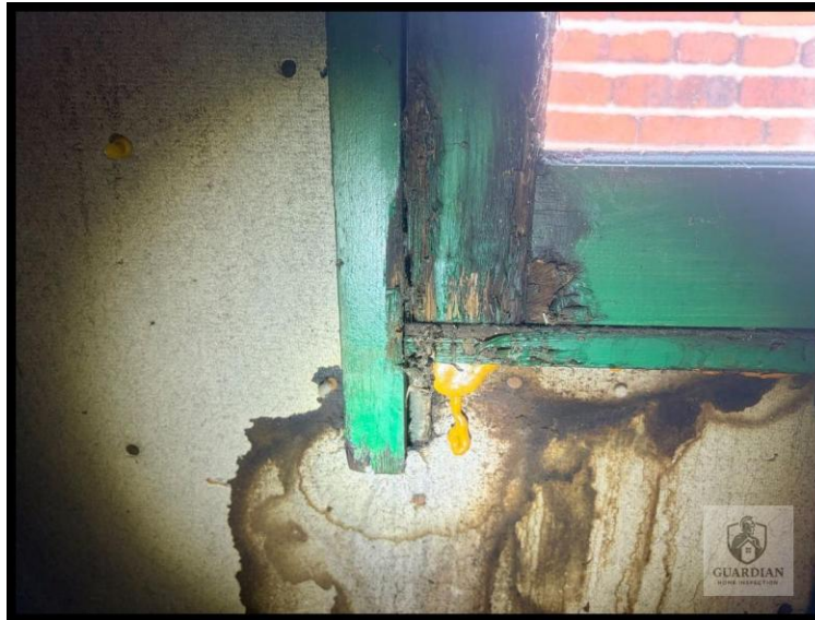
Figure 23: Severe wood rot was observed at an exterior window frame/sill, with peeling paint and moisture staining consistent with active or prior water intrusion.
