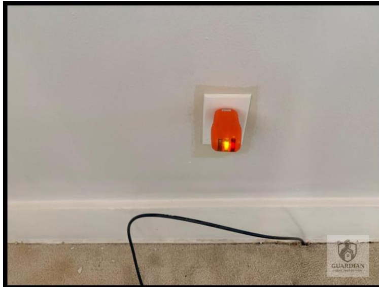
Figure 11: Multiple receptacles in the Living Room and Bedroom indicated open ground conditions and open neutral conditions during testing.
