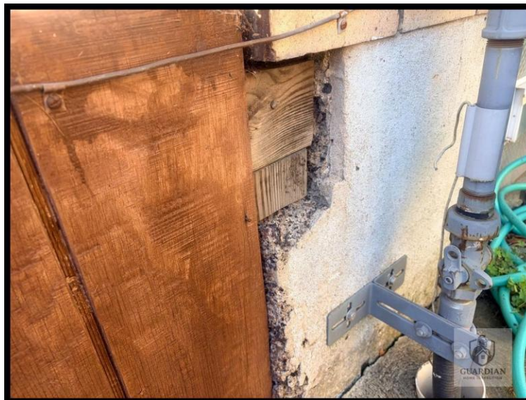
Figure 16: Open gaps and deteriorated mortar/sealant were observed at an exterior brick-to-wood/stucco corner joint.
