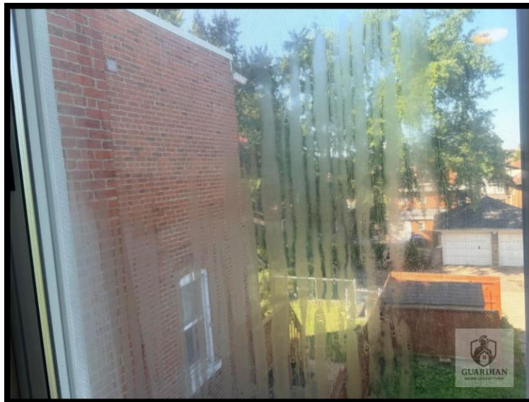
Figure 28: Heavy condensation and water streaking were observed between the window panes in the bedroom, consistent with a likely failed insulated glass seal.
