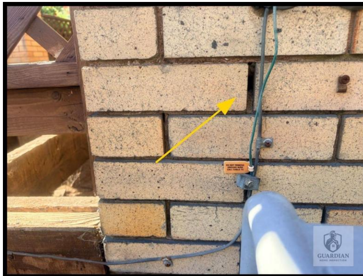
Figure 15: Open gaps and deteriorated mortar/sealant were observed at an exterior brick-to-wood/stucco corner joint.
