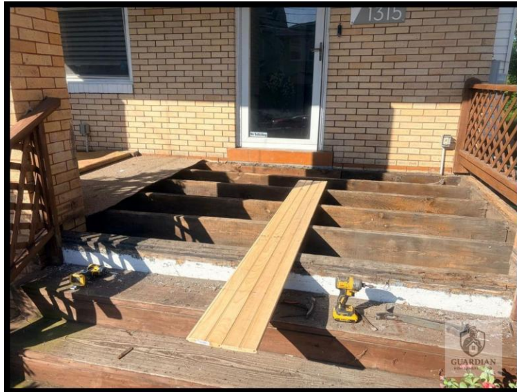
Figure 33: The front porch/deck was under construction at the time of the inspection, and portions of the walking surface were not installed, limiting evaluation of the complete assembly.
