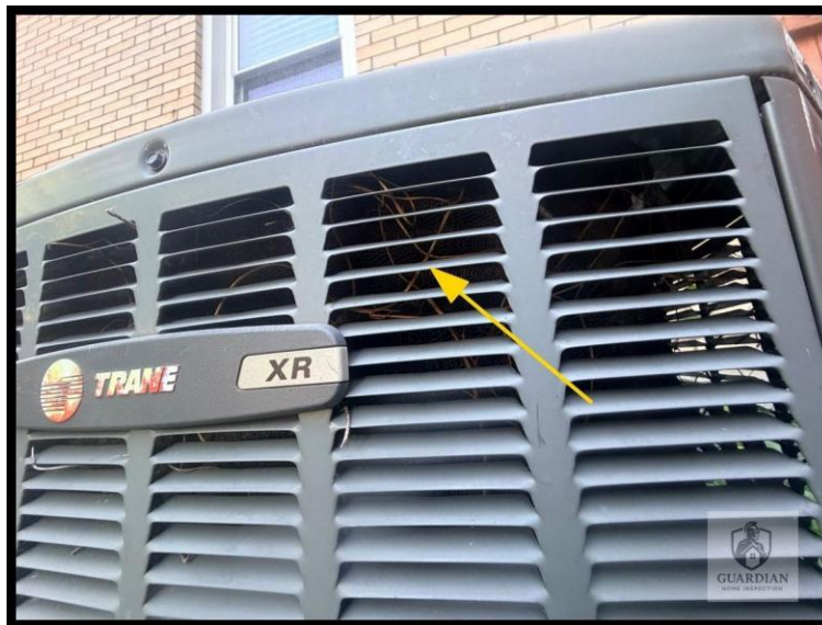
Figure 32: Overgrown vegetation and debris were observed inside and around the outdoor A/C condenser, restricting airflow through the coil area and limiting service access.
