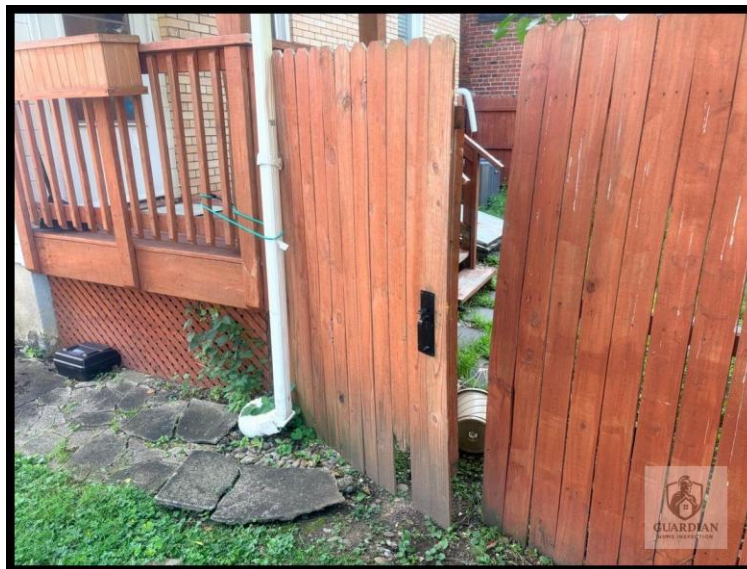
Figure 20: The exterior privacy gate was observed to be damaged and difficult to open/close.
