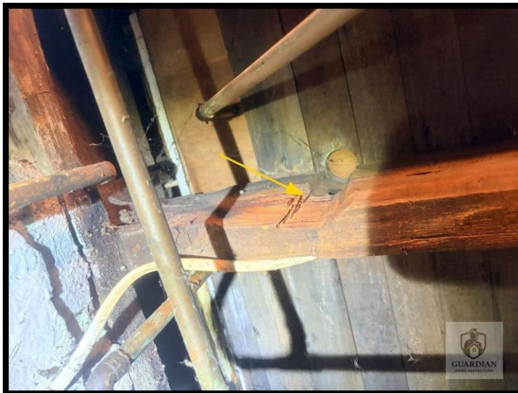
Figure 2: Over-notched and poorly constructed floor joists were observed in the basement.
