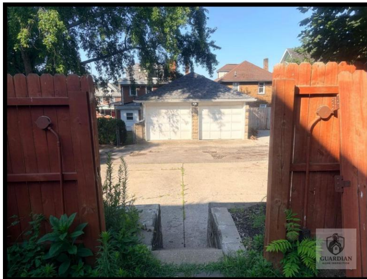
Figure 34: The rear privacy gate was observed to be dismantled at the time of inspection.
