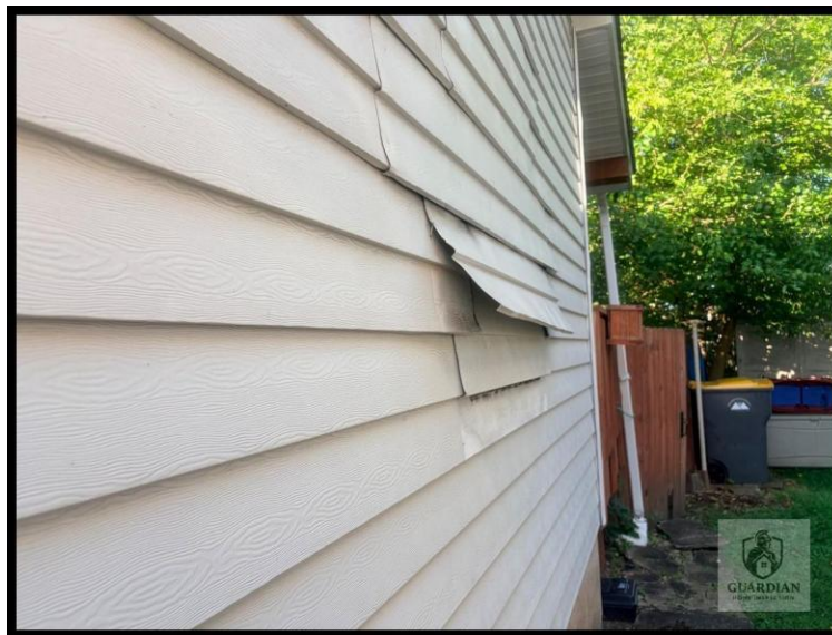
Figure 18: Exterior lap siding was observed to be broken/warped and pulling loose, leaving visible gaps at the exterior wall.
