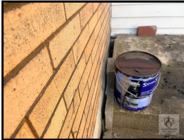
Figure 17: A gap/opening was observed at the base of the exterior wall/brick veneer, leaving an unsealed area at the wall-to-grade/slab interface.
