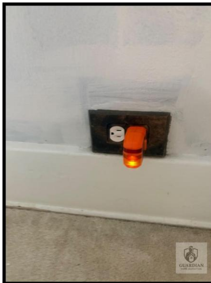
Figure 10: Multiple receptacles in the Living Room and Bedroom indicated open ground conditions and open neutral conditions during testing.
