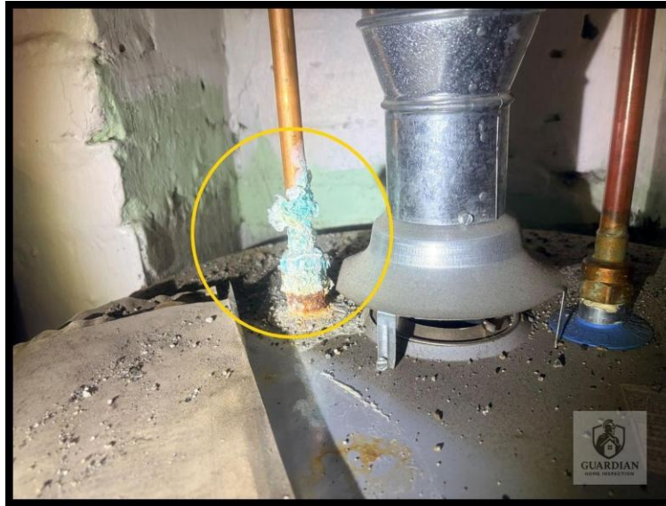
Figure 25: Severe corrosion and mineral buildup were observed on a copper pipe/connection at the water heater in the basement, indicating a possible active or past leak.
