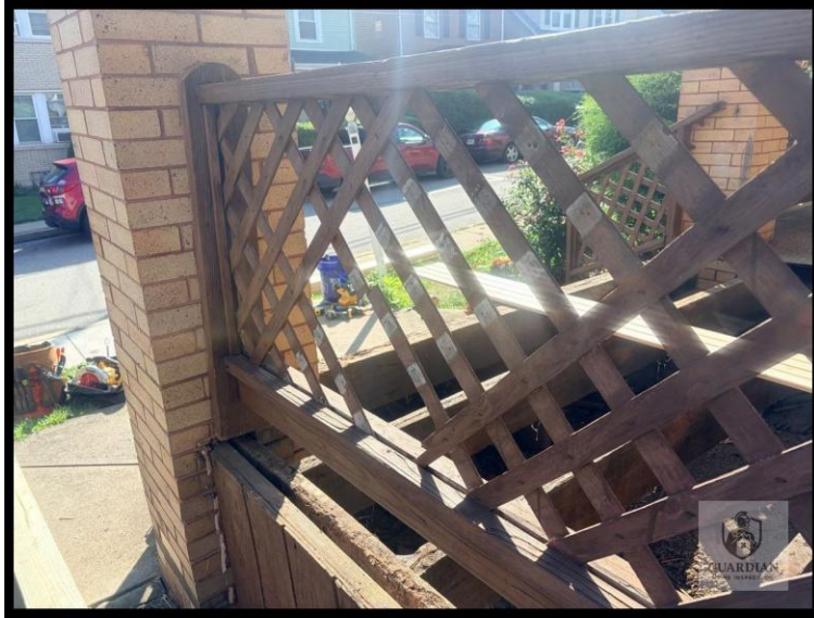
Figure 13: The exterior wood lattice/porch railing was observed to be broken, loose, and deteriorated, with missing/rotted sections.
