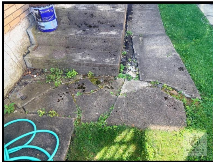
Figure 6: Cracked and broken concrete was observed at the exterior walkway/landing, with vegetation growth through the damaged areas and resulting uneven surfaces.
