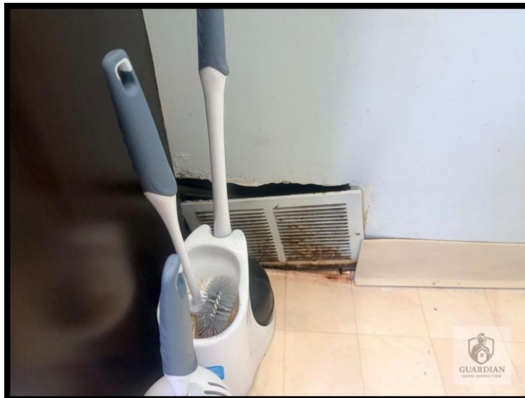
Figure 30: Damaged drywall was observed around the bathroom HVAC return vent, including a visible gap at the wall opening and water staining/rust at the return grille and adjacent baseboard area.
