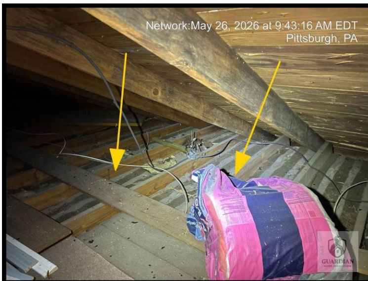
Figure 25: The attic insulation levels were observed to be poor/inadequate in the attic area.
