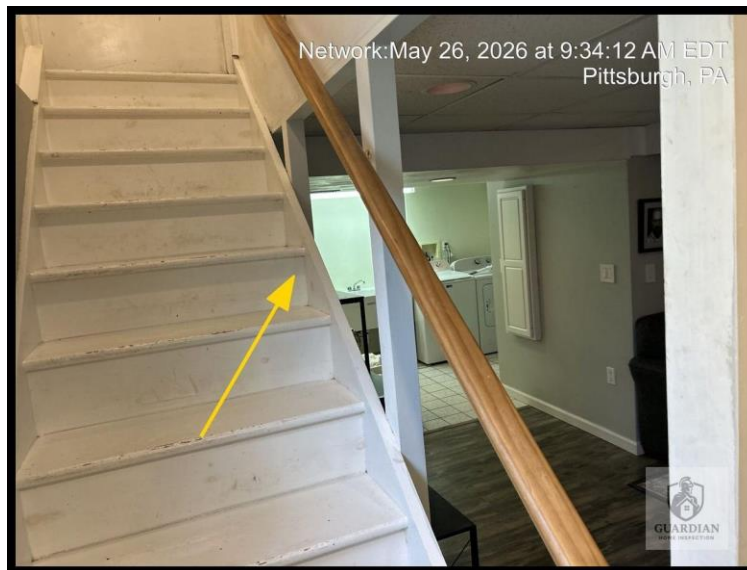
Figure 2: The basement stairway was observed to lack an adequate handrail/rail protection, as shown in the provided photo.
