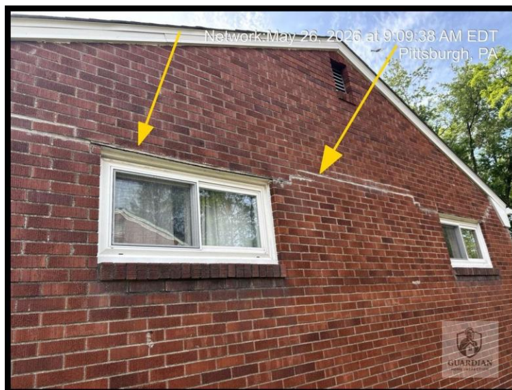
Figure 10: Steel lintels along the right-facing exterior brick wall were observed to be sagging, with associated step cracking and mortar cracking in the surrounding brickwork.
