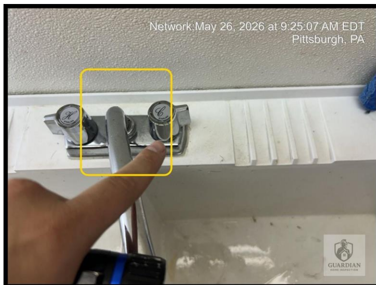
Figure 16: The cold water faucet handle at the basement laundry sink was observed to spin without properly operating the valve.
