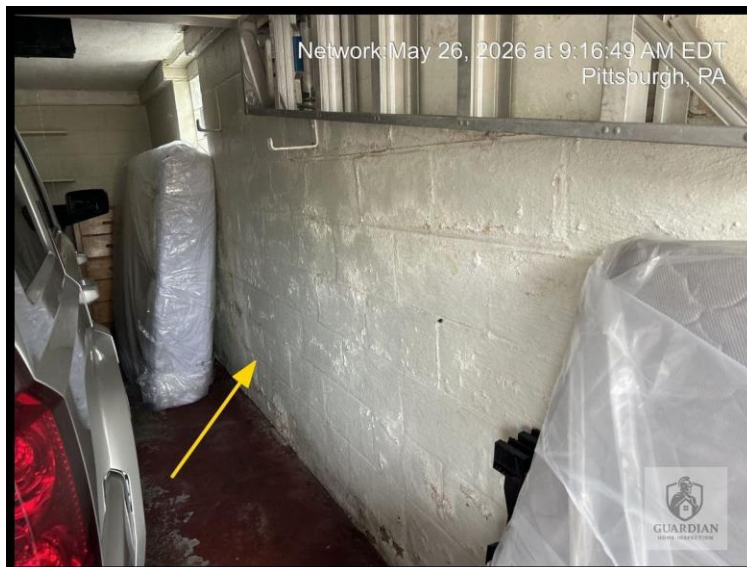
Figure 19: Evidence of moisture intrusion was observed along the right-facing interior garage wall, with visible staining/efflorescence consistent with water migration through the masonry.
