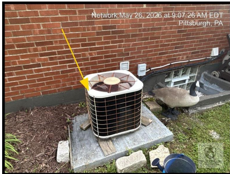
Figure 27: The exterior air conditioning condensing unit appears to be older and, based on its apparent age/condition, is approaching the end of its typical useful life.
