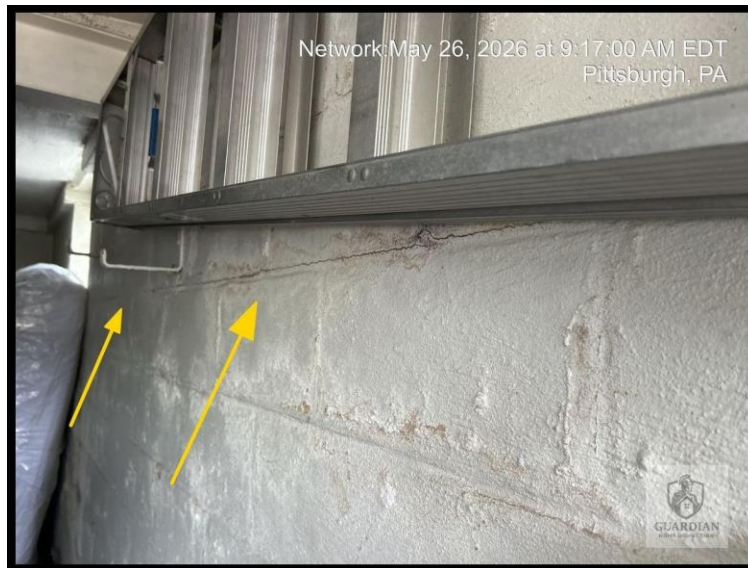
Figure 21: Evidence of hairline, step, and horizontal cracking was noted along the right-facing wall in the garage.
