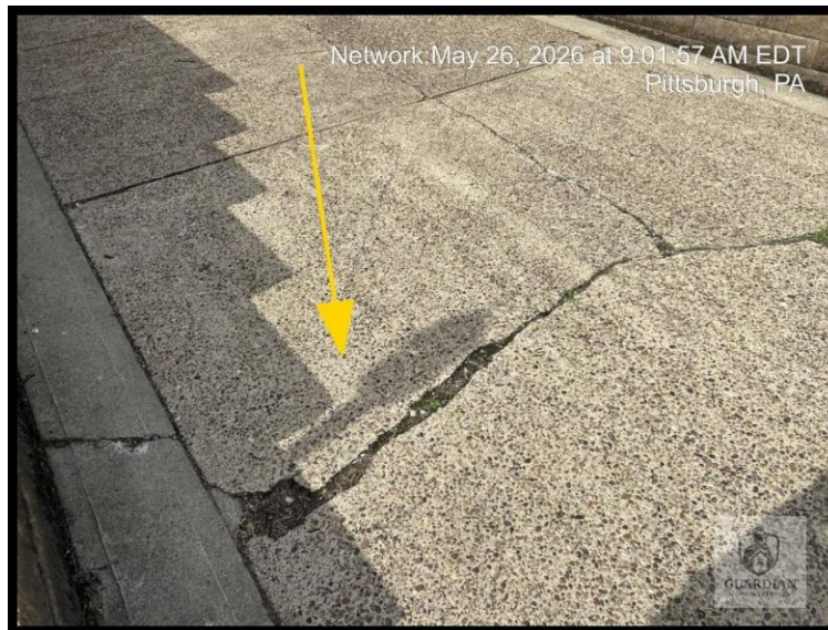
Figure 5: Minor cracking was observed in the concrete driveway.
