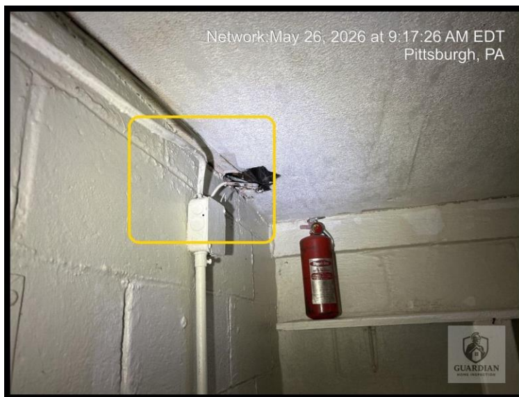
Figure 4: A visible gap/opening was observed along the garage ceiling, which can compromise the required fire-resistance separation between the garage and adjacent areas.
