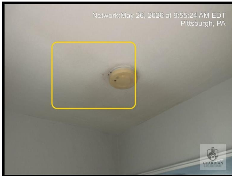
Figure 3: Carbon monoxide protection was not observed in the living space in the hallway at the time of inspection.
