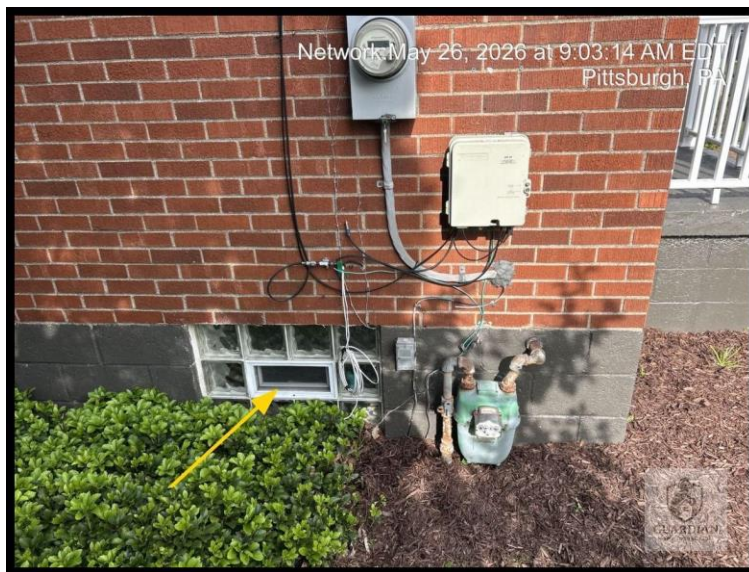
Figure 14: The left-facing exterior electrical outlet was observed to be loose from the wall.
