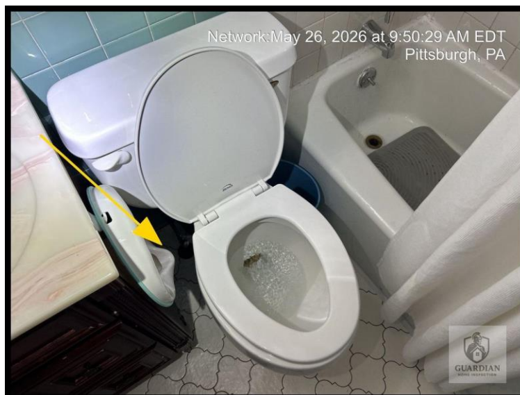
Figure 18: The hallway bathroom toilet was observed to be loose at the floor.
