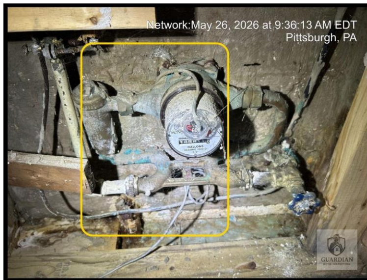
Figure 23: Corrosion was observed on the fittings and waterlines along the front-facing basement wall.
