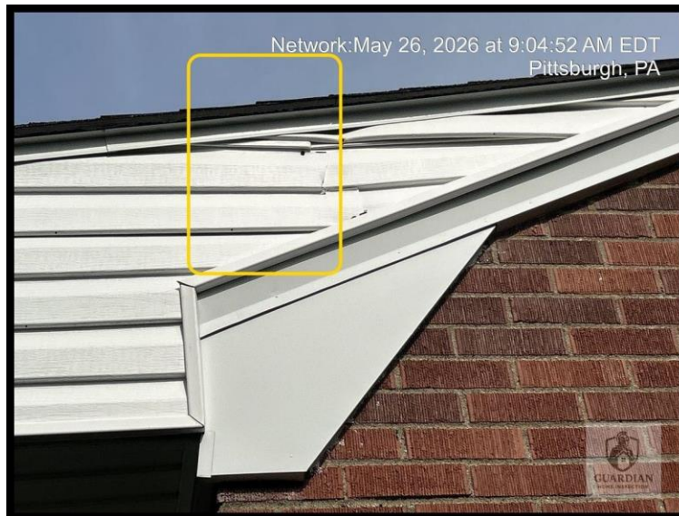
Figure 9: Damaged exterior siding was observed along the left-facing exterior wall.
