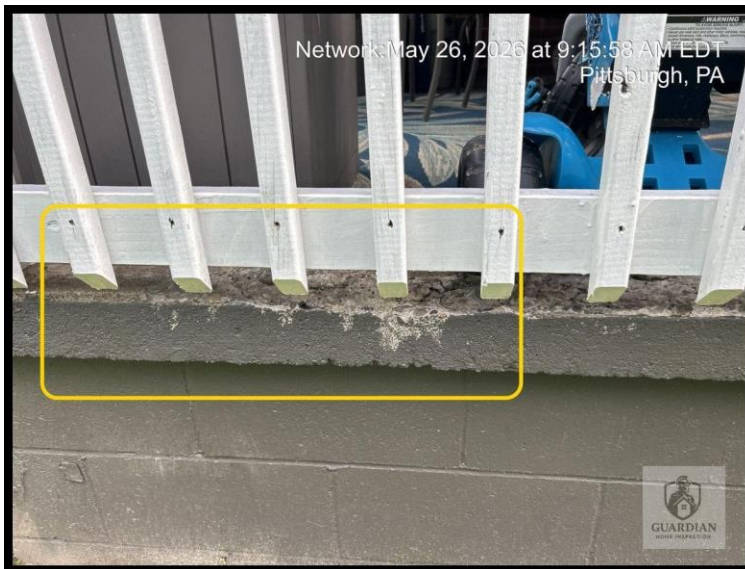
Figure 11: Minor surface spalling/falling was observed along the rear concrete porch edge.
