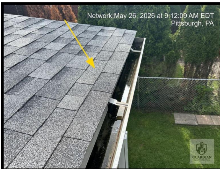
Figure 12: The rear-facing gutter run at the roofline lacked adequate slope, evidenced by standing water observed in the gutter.
