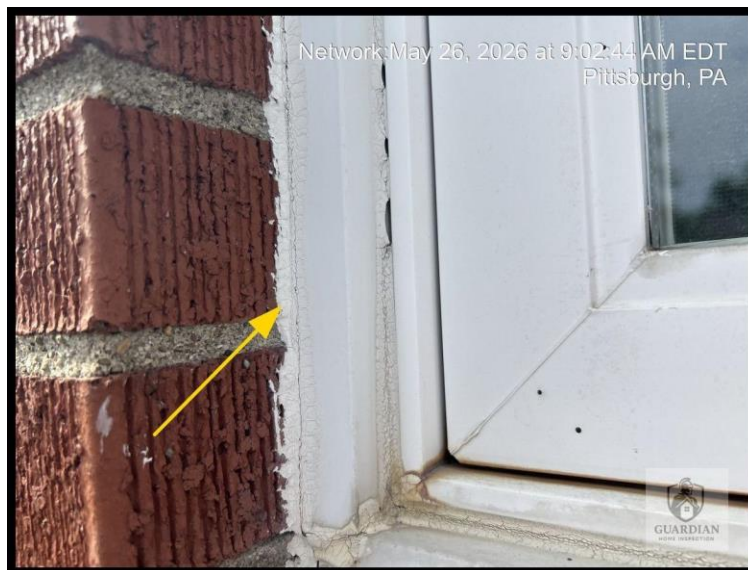
Figure 8: Exterior window and door frame joints were observed with deteriorated/missing sealant at the trim-to-masonry/frame interfaces.
