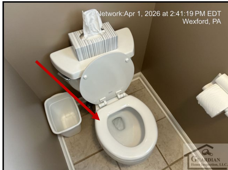
Figure 10 The toilet, in the 2nd floor primary bathroom, is loose from the floor.
