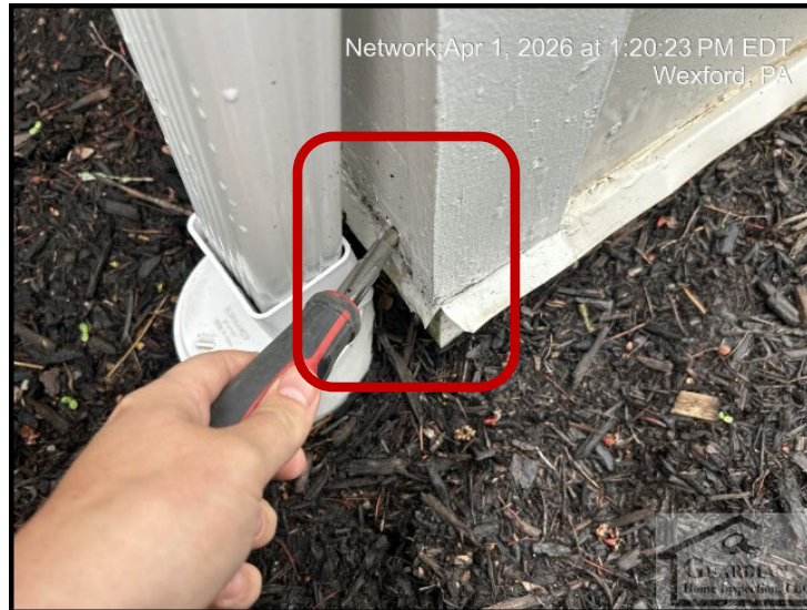
Figure 5 An area of moderately rotted siding, along the front facing exterior wall, was noted.
