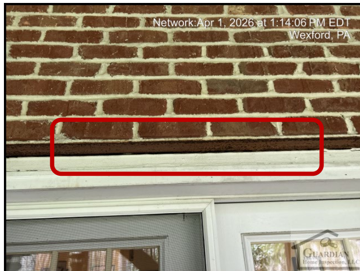
Figure 2 Several of the steel lintels, installed to support brick above door or window openings, are beginning to rust
