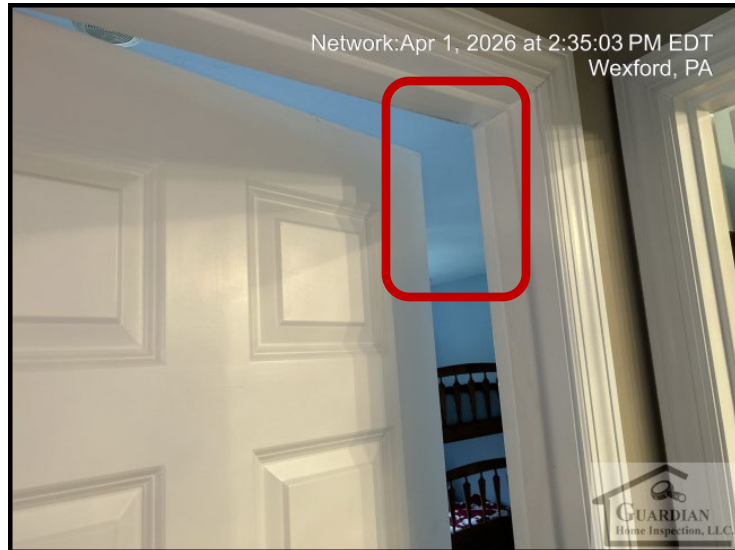
Figure 9 The 2 nd floor bedroom door does not open/close smoothly and should be trimmed or adjusted as necessary.
