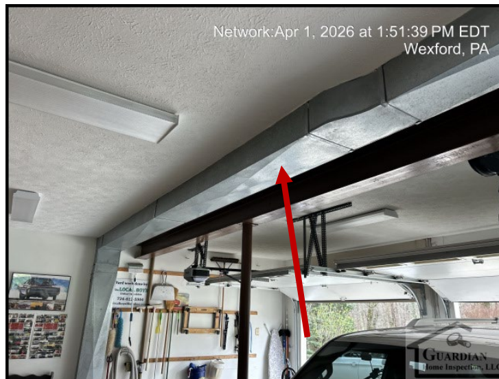
Figure 6 The supply ductwork in the garage should be insulated to prevent unnecessary heat/cooling loss.
