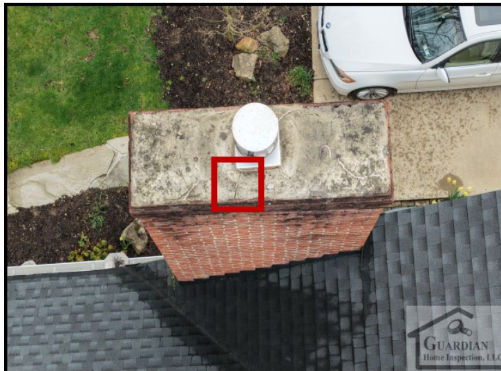
Figure 12 The masonry crown, on the chimney, is cracked.
