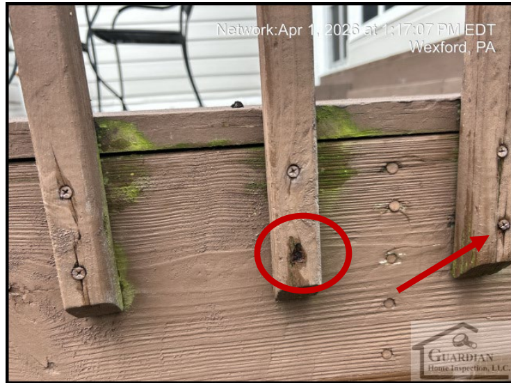
Figure 3 Several of the securing hardware (screws), supporting the vertical balusters on the rear deck, are significantly rusted.
