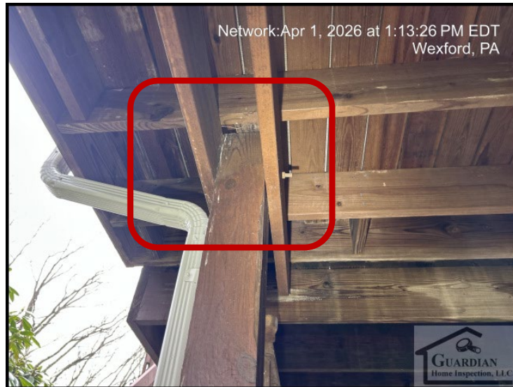
Figure 1 The vertical support posts, on the rear exterior decking, have been poorly connected to the connecting horizontal double header beams
