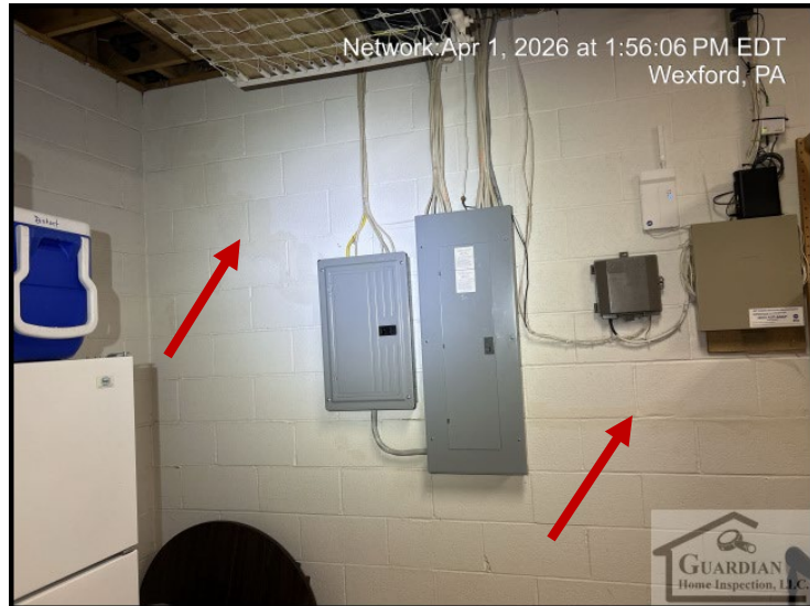
Figure 7 A limited amount of past repairs & horizontal and step cracking was observed along left facing block foundation wall.
