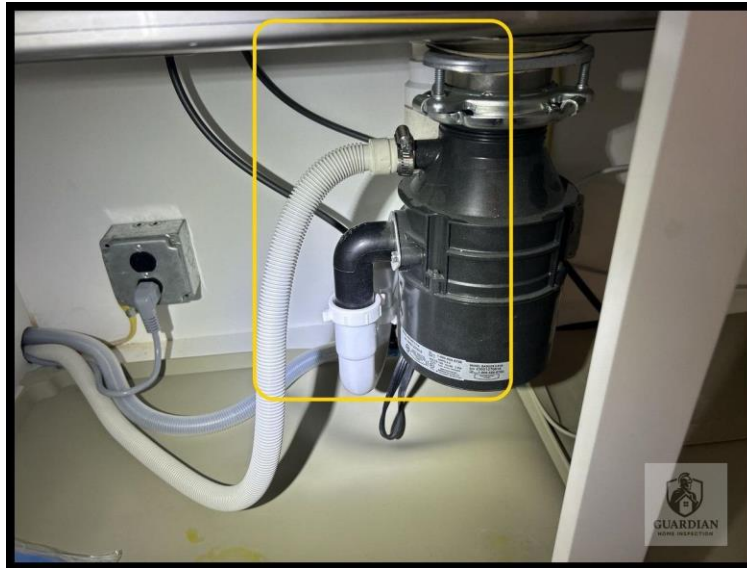
Figure 13: The kitchen waste disposal was observed to operate louder than typical during testing.
