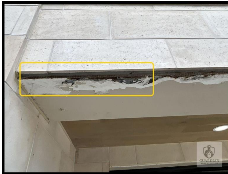
Figure 1: The lintel above the garage door exhibited visible rust staining and minor deterioration/spalling of the adjacent concrete/finish.
