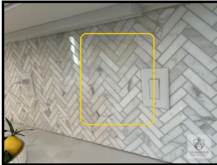
Figure 11: An electrical wall switch located at the kitchen countertop/backsplash area was present, and its function could not be verified at the time of inspection.
