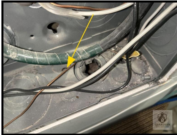
Figure 7: In the Lower Utility Room, the electrical panel cabinet had missing open knockouts.
