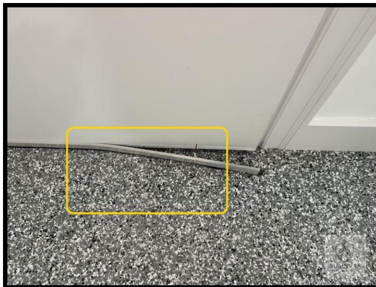
Figure 14: The bottom trimming component/door sweep at the door leading to the lower utility room in the garage was observed damaged and partially detached.
