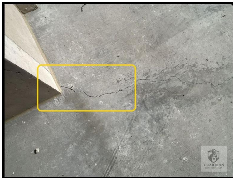
Figure 2: Minor hairline cracking was observed along the front-facing concrete sidewalk.
