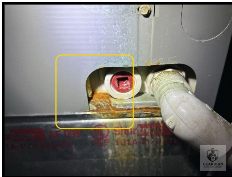
Figure 4: In the 3rd Floor Utility Room, the air-conditioning overflow knockout was observed actively leaking at the air handler cabinet.
