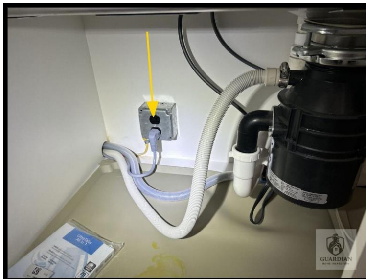
Figure 10: At the kitchen sink cabinet, the dishwasher drain hose was observed without a high loop secured to the underside of the countertop.
