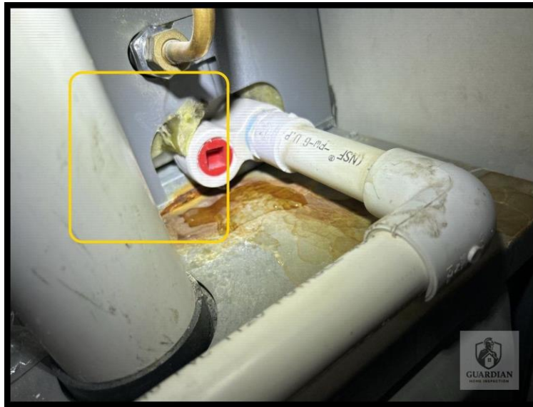
Figure 5: In the Lower Utility Room, water staining and active moisture were observed at the air conditioner overflow condensate knockout, with leakage running along the basement furnace cabinet.
