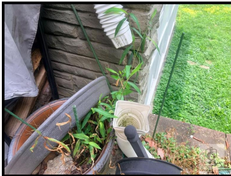
Figure 16: A downspout extension was observed to be disconnected and/or damaged at the base, resulting in roof runoff discharging near the foundation.
