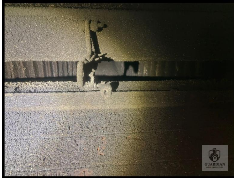
Figure 39: Heavy soot buildup was observed at the wood-burning fireplace in the Living Room.
