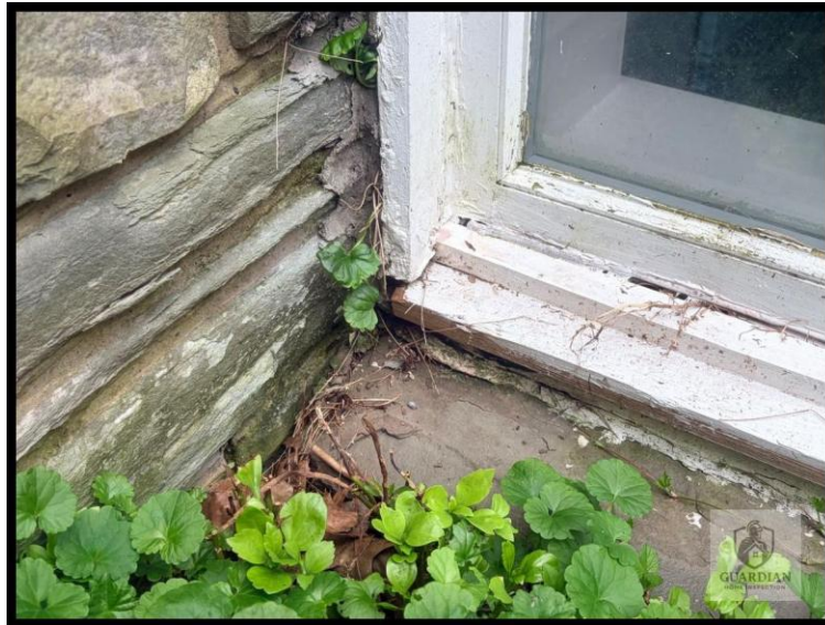
Figure 17: Deteriorated wood and peeling paint were observed at exterior window trim/sills, indicating moisture exposure and inadequate sealing.
