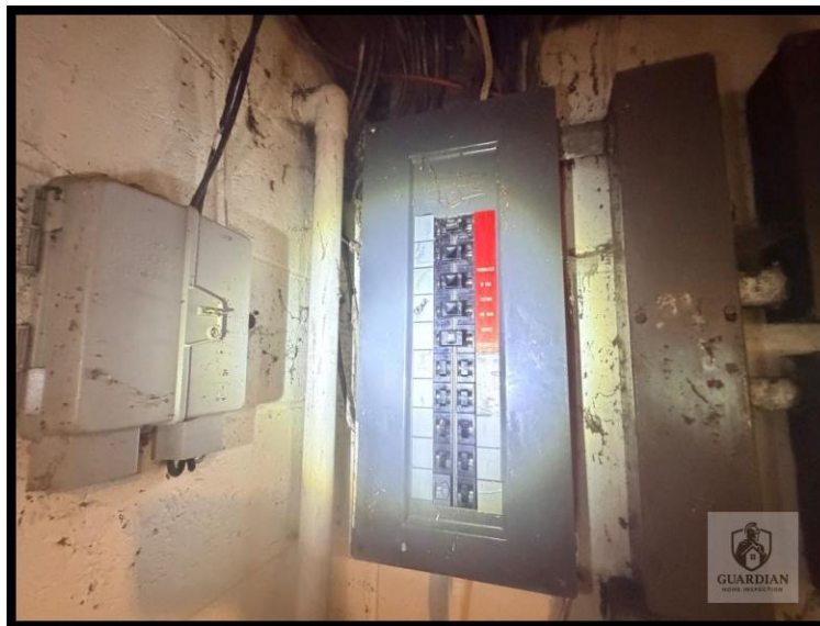
Figure 6: Pushmatic-style breakers were observed at the main electrical panel and the subpanel in the basement.
