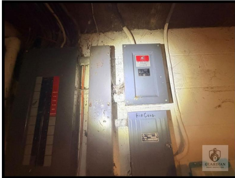
Figure 7: Pushmatic-style breakers were observed at the main electrical panel and the subpanel in the basement.
