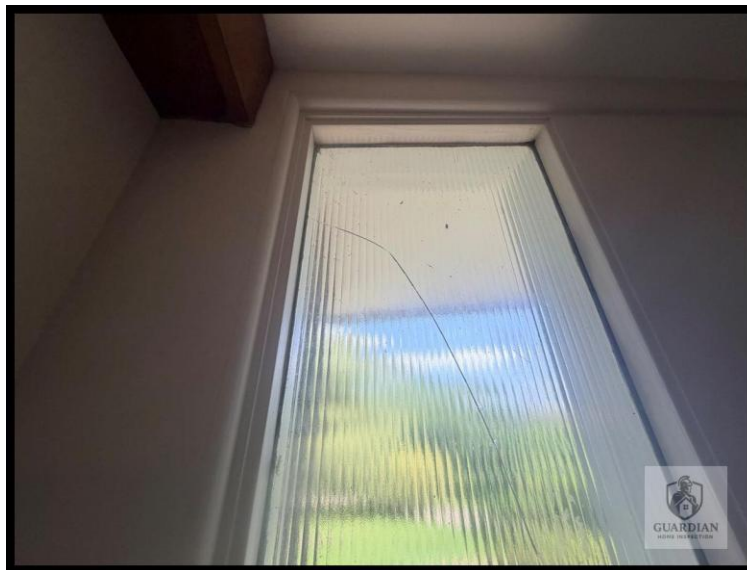
Figure 26: Cracked window glass was observed beside the main entry door on the first floor.
