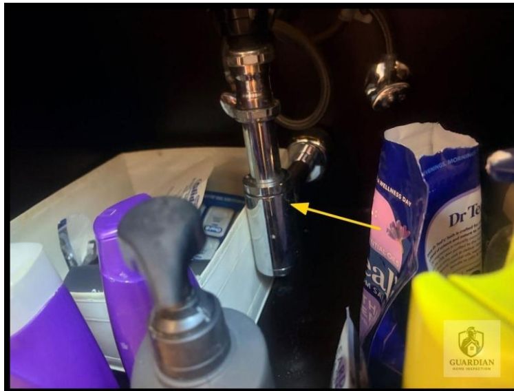
Figure 33: No P-trap was observed installed under the master bathroom sink drain piping at the time of inspection.
