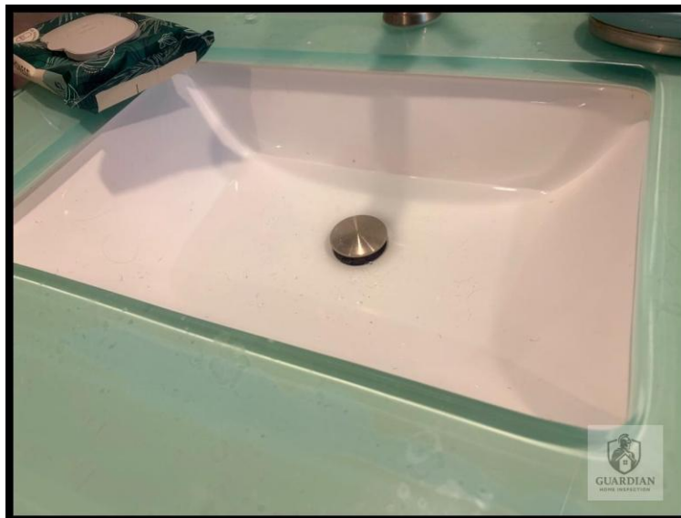
Figure 34: The master bathroom sink was observed to drain very slowly at the time of inspection.
