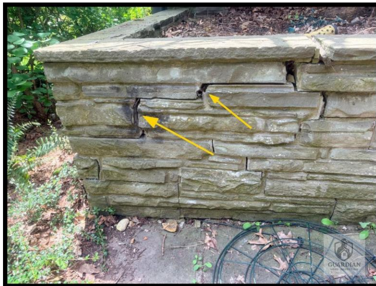
Figure 10: Cracked and separating stone veneer/masonry was observed at the exterior, with displaced blocks and open joints consistent with movement.
