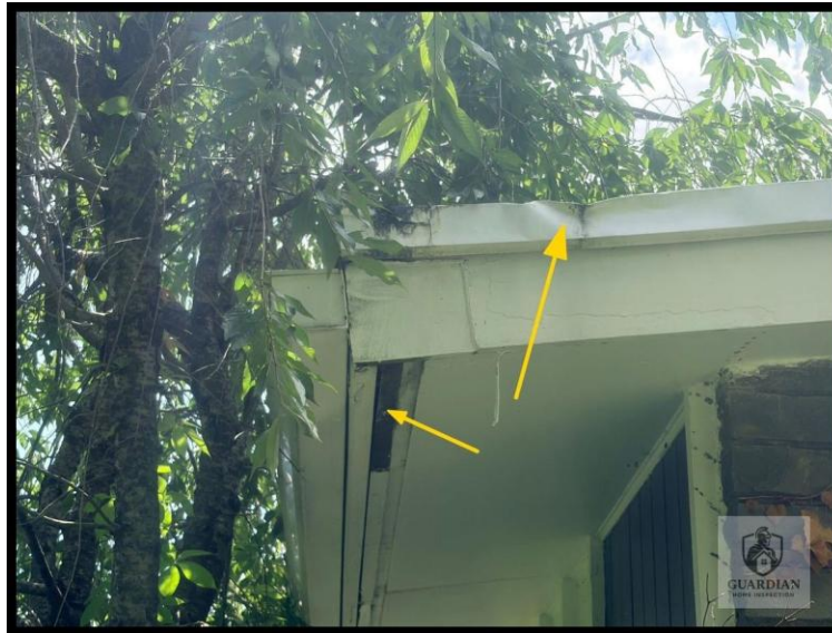
Figure 13: Damage and missing wood were observed at the fascia/soffit along the roof edge at the exterior.
