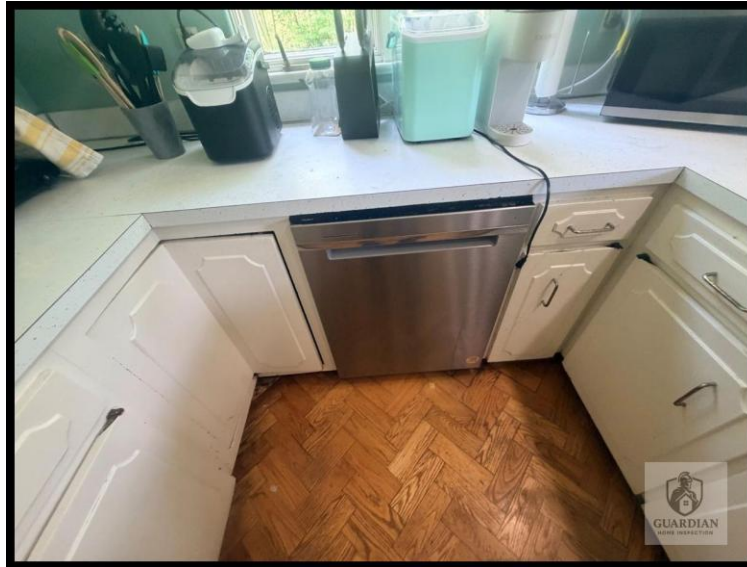
Figure 27: The kitchen dishwasher did not operate at the time of inspection.
