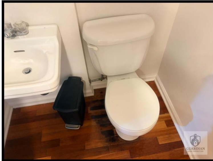
Figure 23: The toilet in the basement bathroom was observed to be loose at the base.
