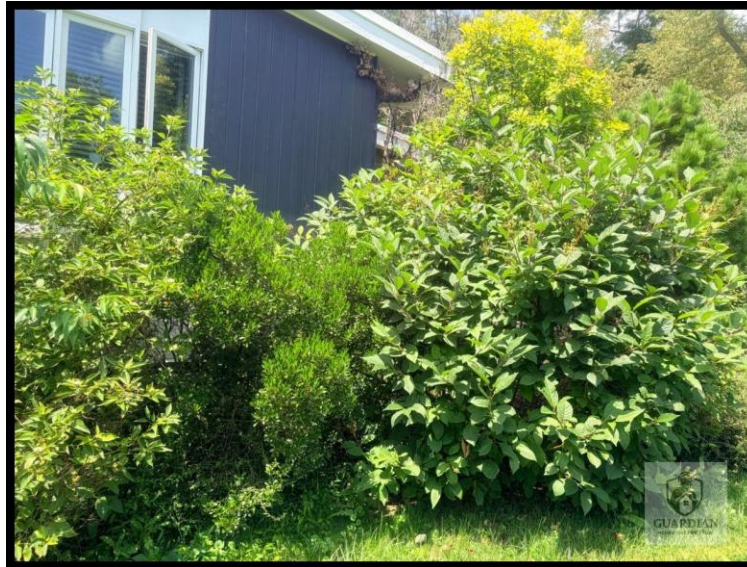
Figure 29: Overgrown shrubs and vegetation were observed in contact with the exterior siding and adjacent to windows.
