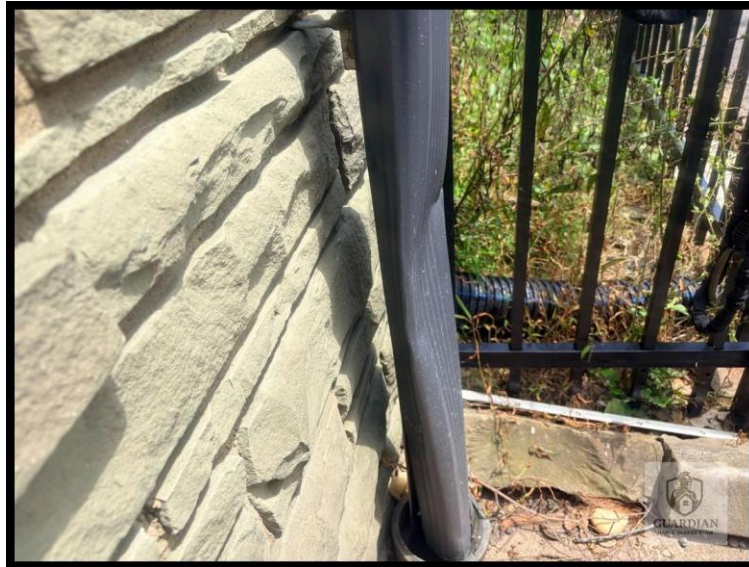
Figure 31: Damage was observed at an exterior downspout, which may restrict or reduce proper gutter drainage.
