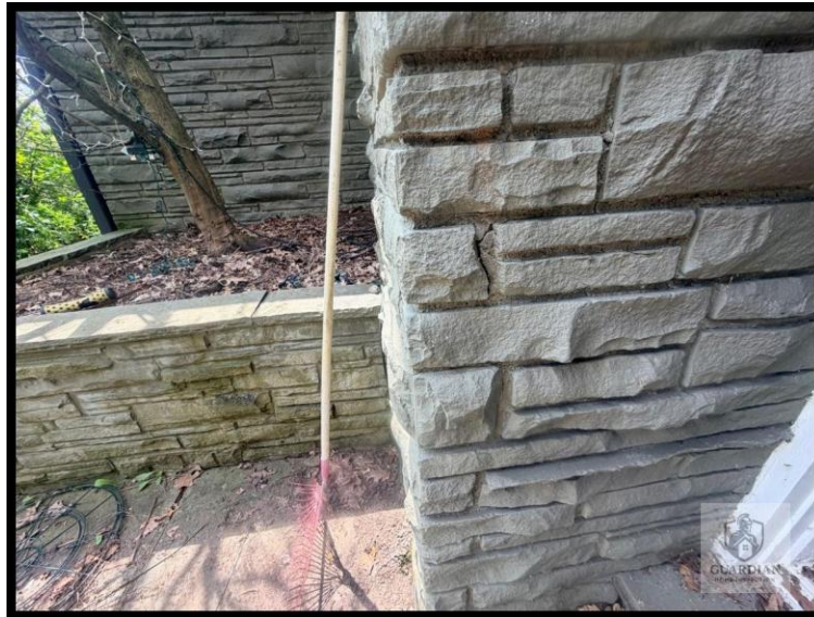
Figure 11: Cracked and separating stone veneer/masonry was observed at the exterior, with displaced blocks and open joints consistent with movement.
