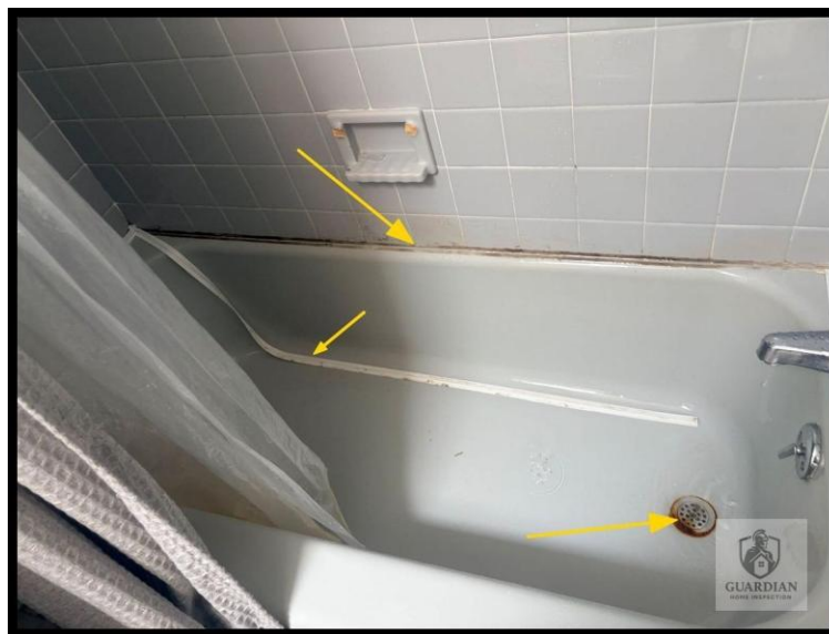
Figure 36: Missing and deteriorated caulk/trim with staining was observed at the bathroom tub surround, and the tub drain was noted to be slow draining.
