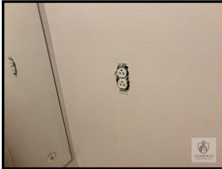
Figure 5: GFCI protection was not present for receptacle(s) in the basement bathroom.
