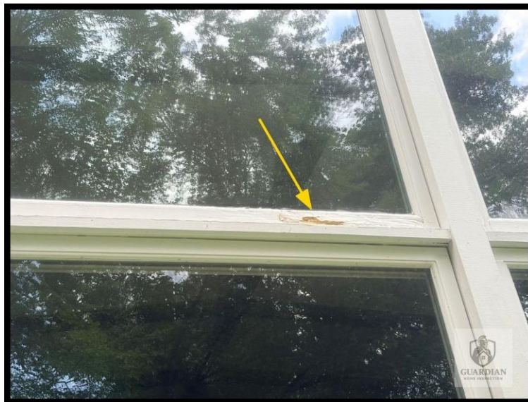
Figure 18: Deteriorated wood and peeling paint were observed at exterior window trim/sills, indicating moisture exposure and inadequate sealing.
