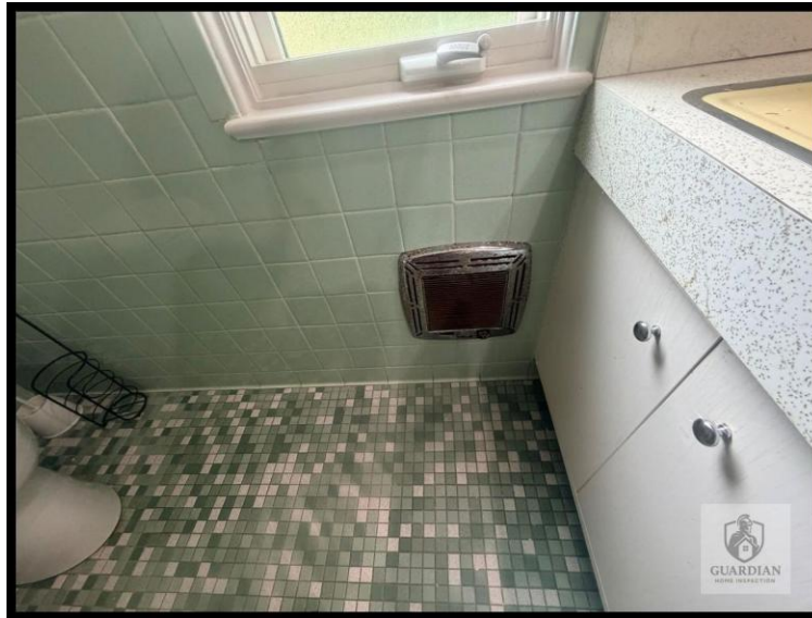
Figure 21: The bathroom wall-mounted heater was observed to be non-operational at the time of inspection.
