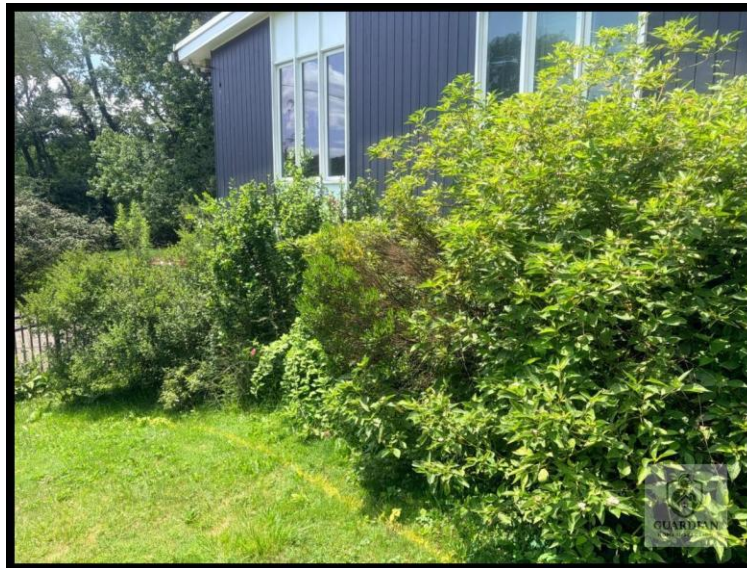
Figure 28: Overgrown shrubs and vegetation were observed in contact with the exterior siding and adjacent to windows.
