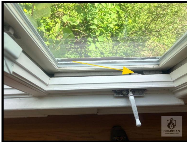
Figure 25: A bedroom window operator linkage was observed to be broken/disconnected at the time of inspection.
