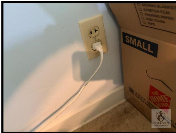
Figure 2: Multiple ungrounded electrical receptacles were observed in the Living Room, Family Room, and Bedroom(s).
