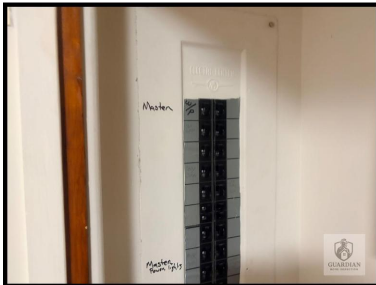
Figure 8: Pushmatic-style breakers were observed at the main electrical panel and the subpanel in the basement.
