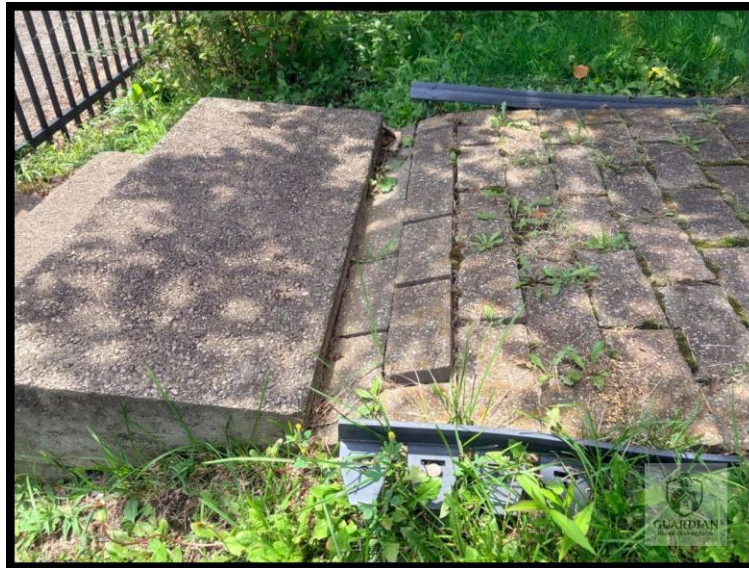
Figure 9: The exterior paver walkway was observed to be uneven and deteriorated, with gaps between pavers and vegetation growth.
