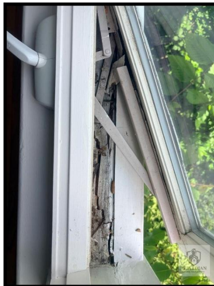
Figure 20: Significant wood rot and material deterioration were observed at the exterior window frame/sill at the opening.
