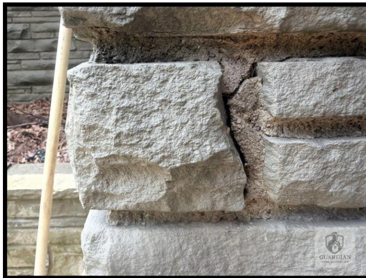
Figure 12: Cracked and separating stone veneer/masonry was observed at the exterior, with displaced blocks and open joints consistent with movement.
