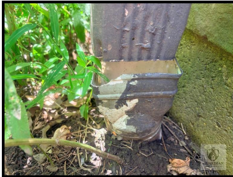
Figure 15: A downspout extension was observed to be disconnected and/or damaged at the base, resulting in roof runoff discharging near the foundation.
