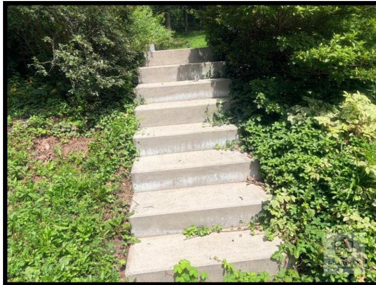
Figure 1: A handrail was not observed at the exterior steps.
