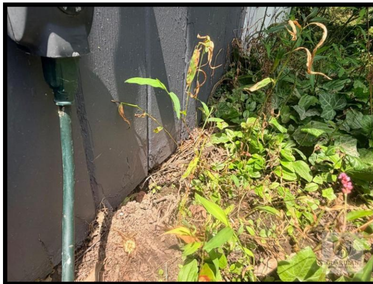
Figure 30: Vegetation and soil were observed in direct contact with the exterior wall.
