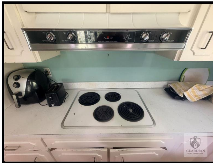
Figure 38: Only one burner on the electric cooktop was observed to function at the time of inspection in the kitchen.
