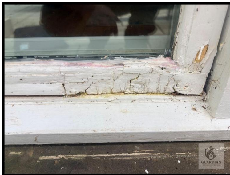
Figure 14: Peeling paint and deteriorated wood were observed at the exterior window sill/trim, indicating possible moisture damage.
