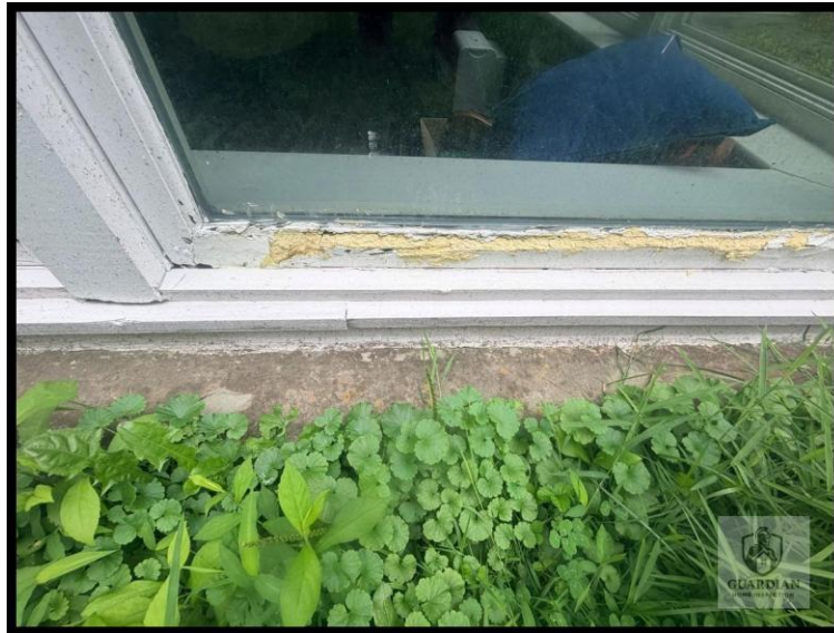
Figure 19: Deteriorated wood and peeling paint were observed at exterior window trim/sills, indicating moisture exposure and inadequate sealing.
