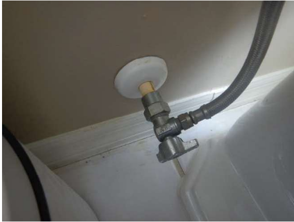
Plumbing – Toilet Supply
