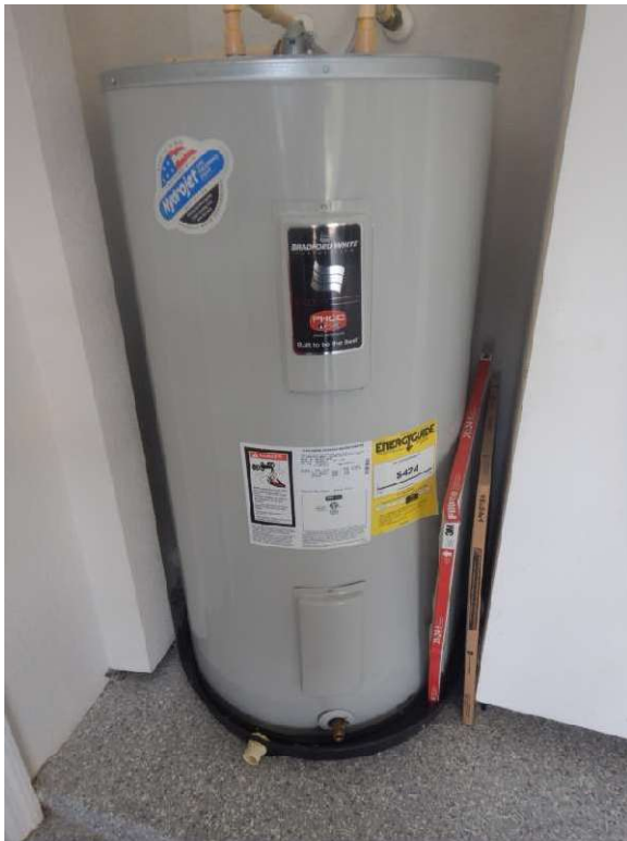
Plumbing – Water Heater
