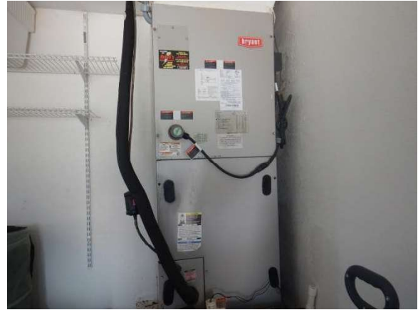
HVAC – Split System
