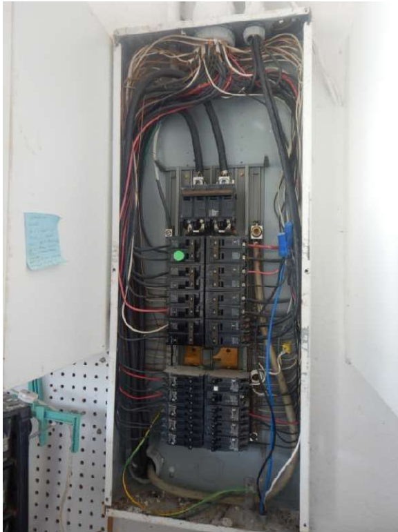
Electric – Main Panel 200A CB
