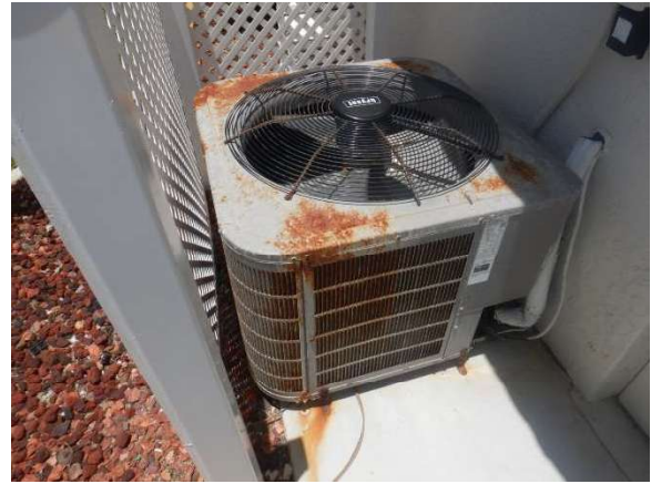
HVAC – Split System
