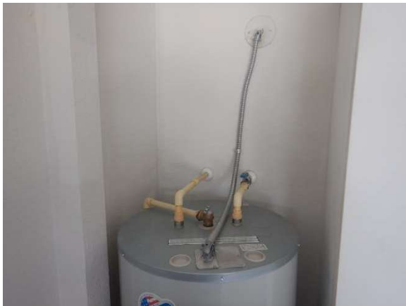
Plumbing – Water Heater
