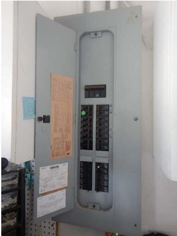
Electric – Main Panel Siemens
