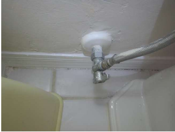
Plumbing – Toilet Supply
