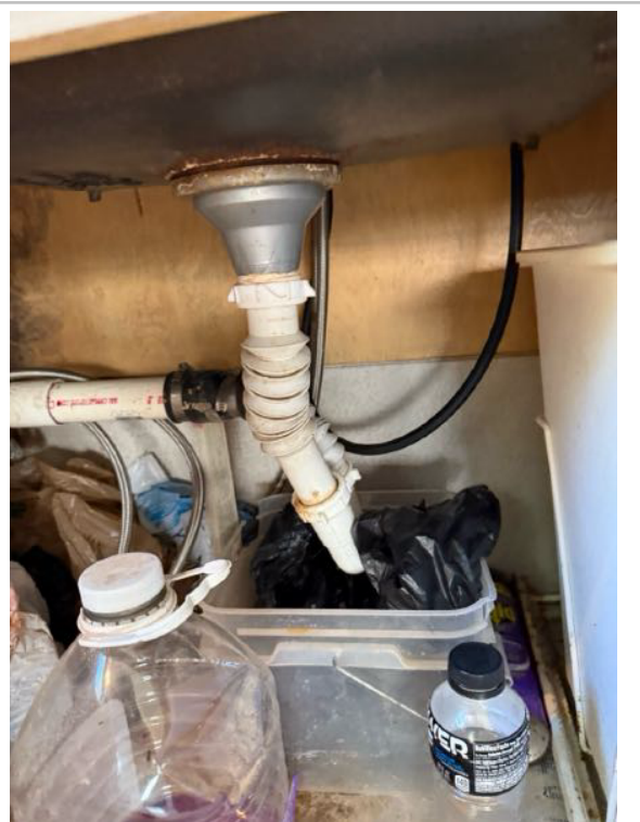
Flex pipe at guest apt. sink drain line
