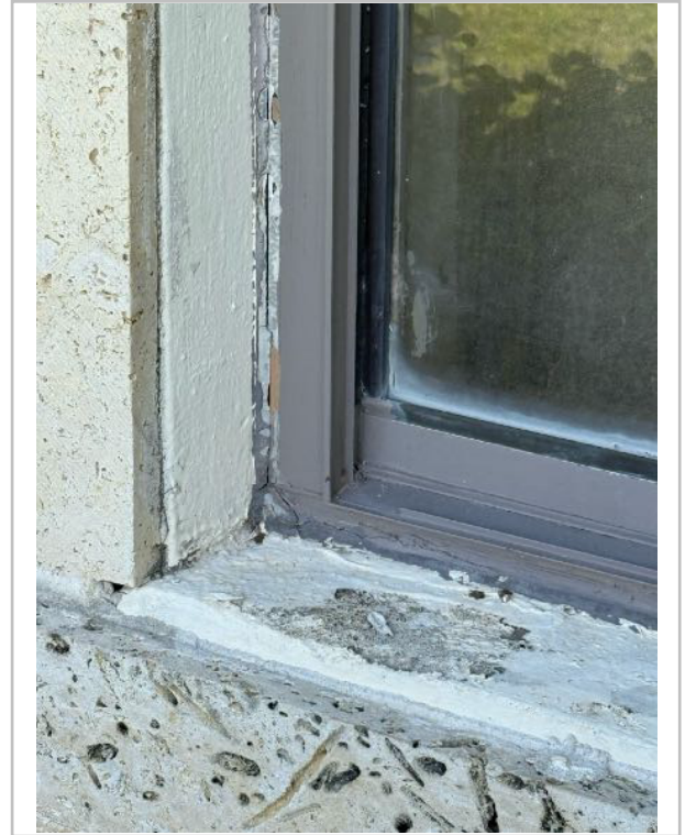
Ex. of voids in window caulking
