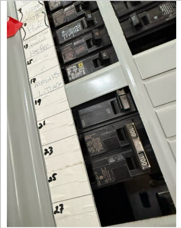
Breaker obstructed in Siemens panel
