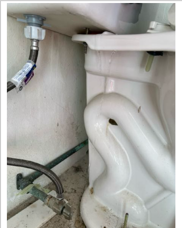
Leak at store room toilet
