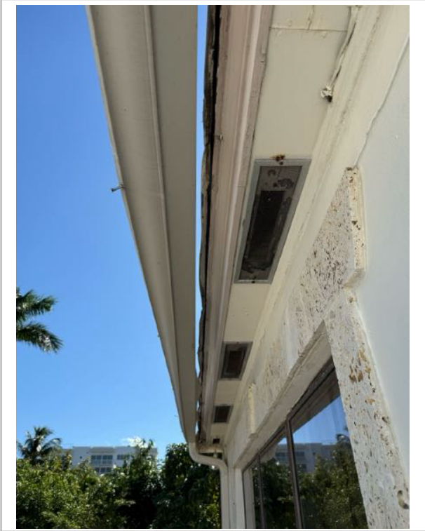
Example of damage to gutter
