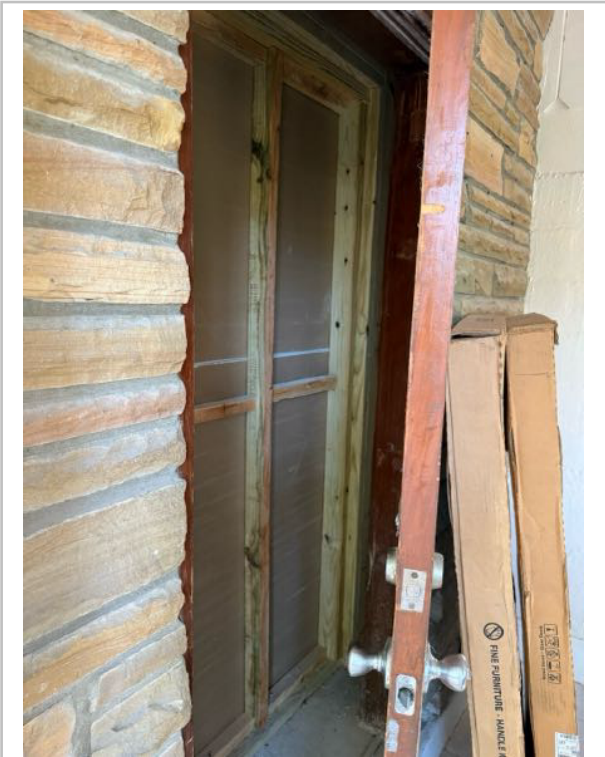
Open wall cavity at guest apartment
