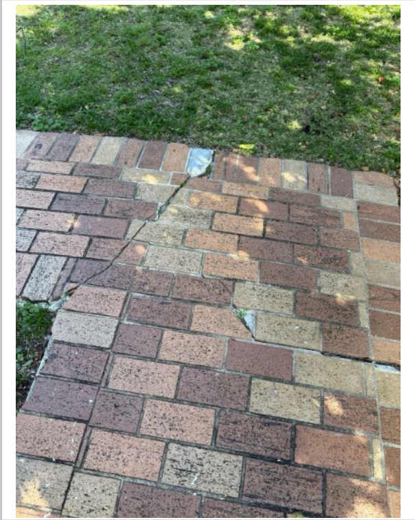
Example of cracks to walkway
