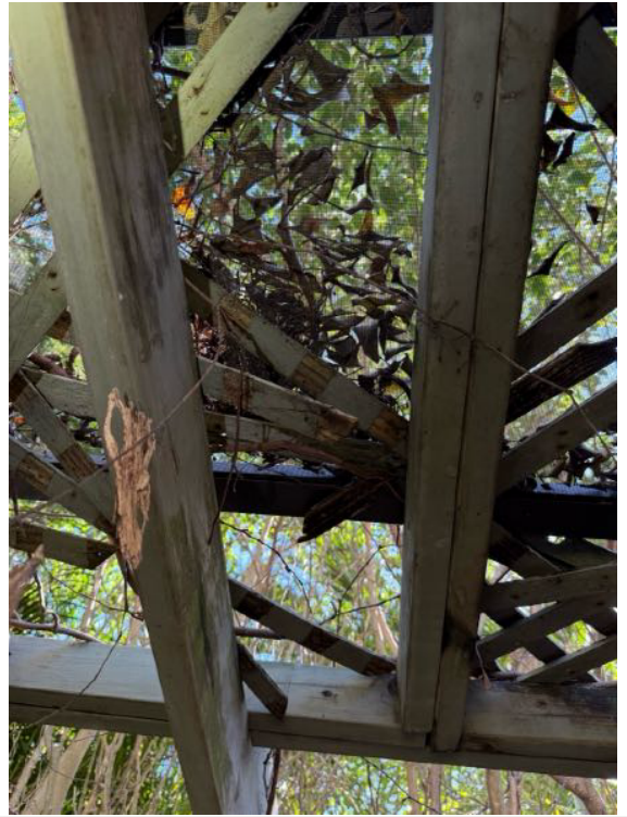
Example of damaged wood at pergola
