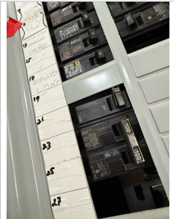
Breaker obstructed guest apt. panel
