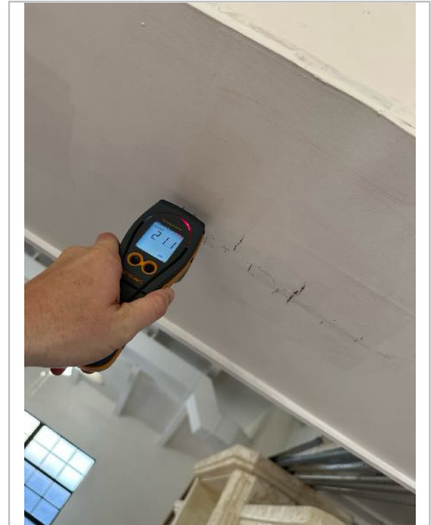
Roof leak over kitchen guest apartment
